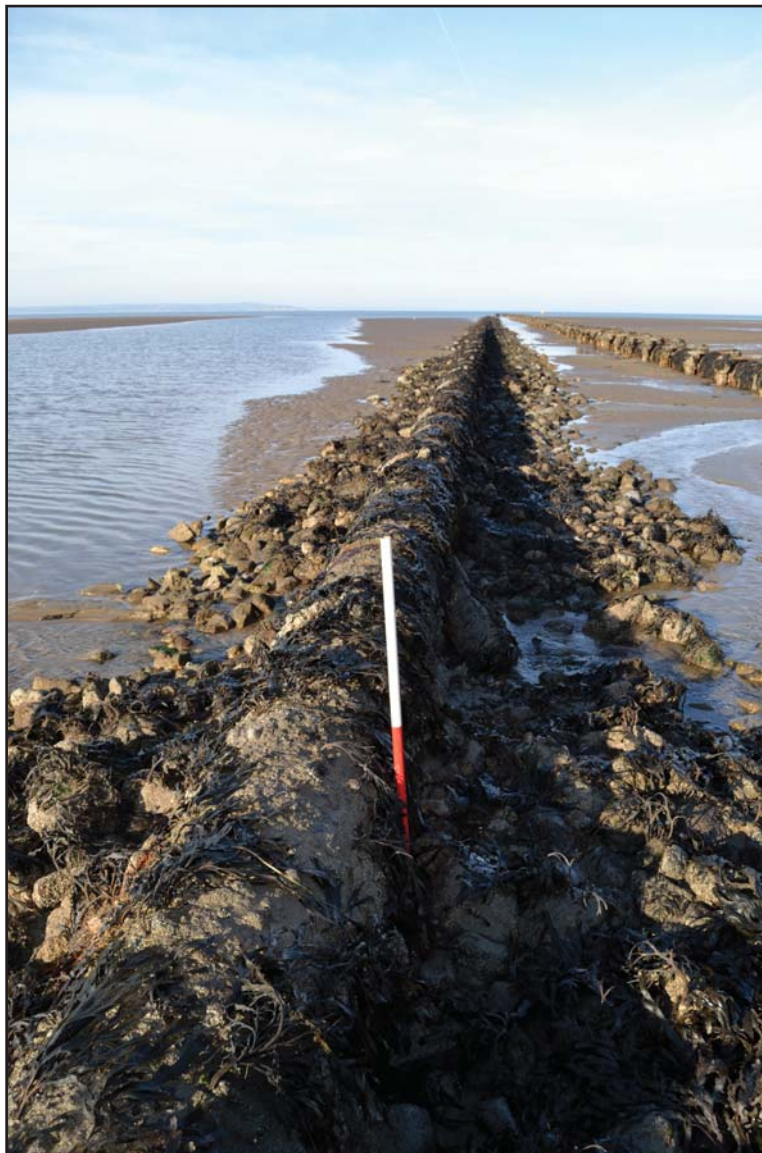
Plate 06: Material collecting around the 1845 pipe view to sea; scale: 1x1m (archive reference: G2600_014).
