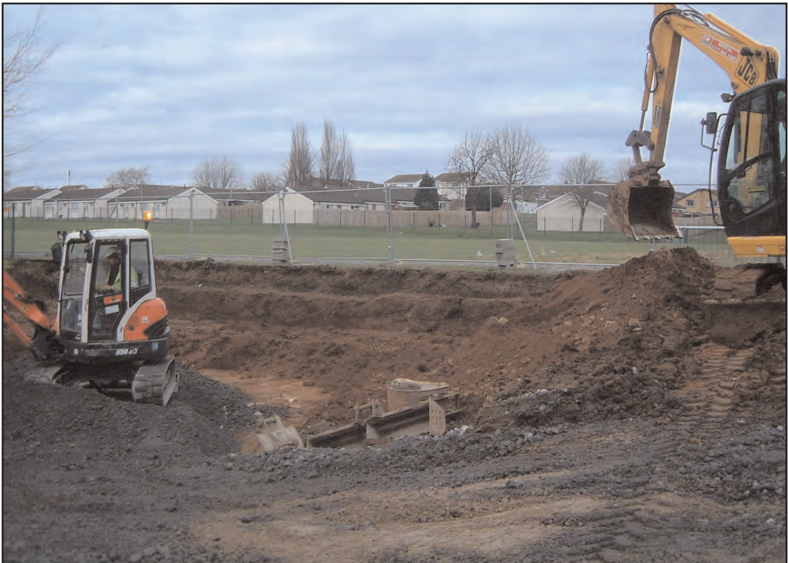
Plate 4 View north west showing stepped 2m high section at the northern limit of the excavation
