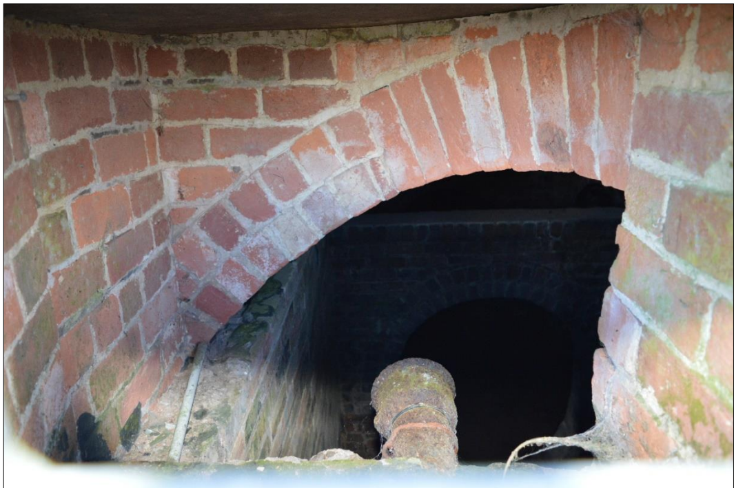
Fig. 7 The access to the tank at the base of the west elevation. Photo CPAT 4602-0007
