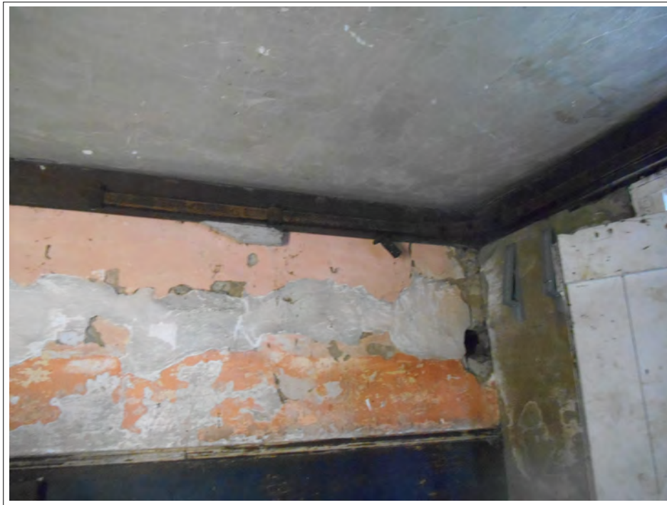
Plate 5. Detail of door track/slide - no longer in use
