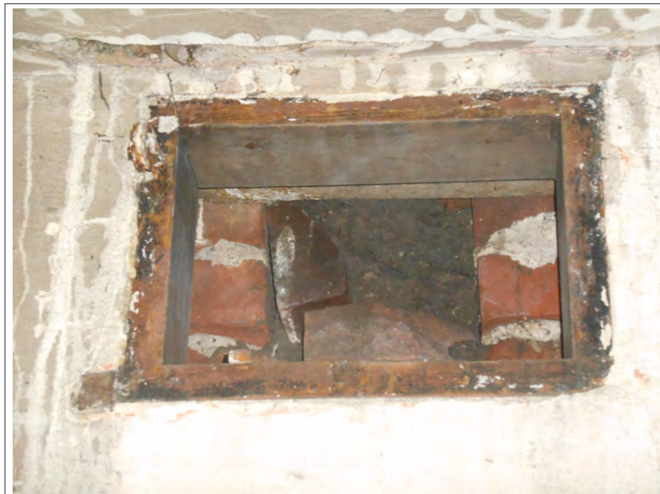
Plate 16. Blocked vent, west facing wall.
