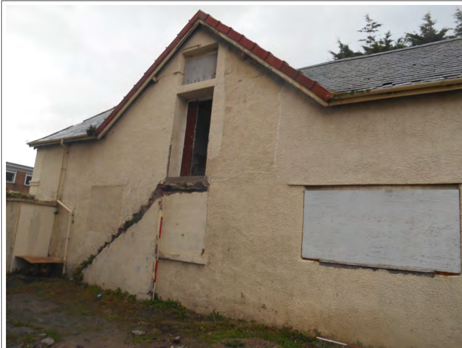
Plate 39. Detail of first floor door and exterior stair case, east facing wall. Scale 2m
