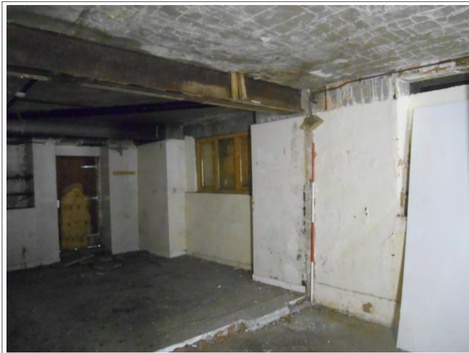
Plate 8. East facing wall. 1960's Window subsequently repaired. North facing wall with back entrance. Not original. Scale 2m
