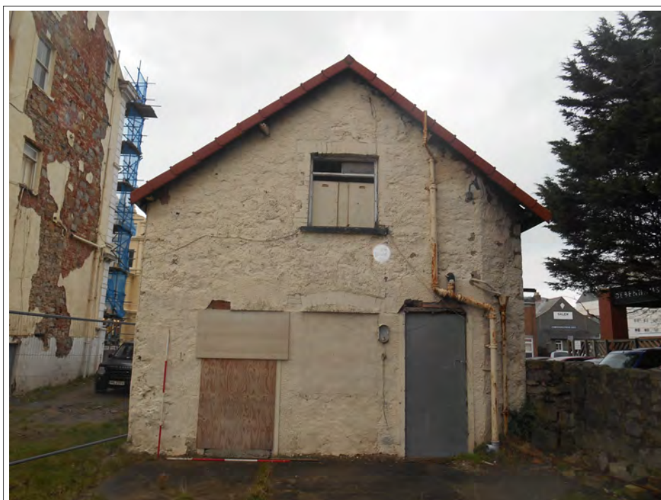
Plate 24. View of back entrance. Windows and doors are not original and demonstrate a number of alterations over time. 1960's hoods. First floor window with reveal toothed brick effect. Scales 2 x 2m
