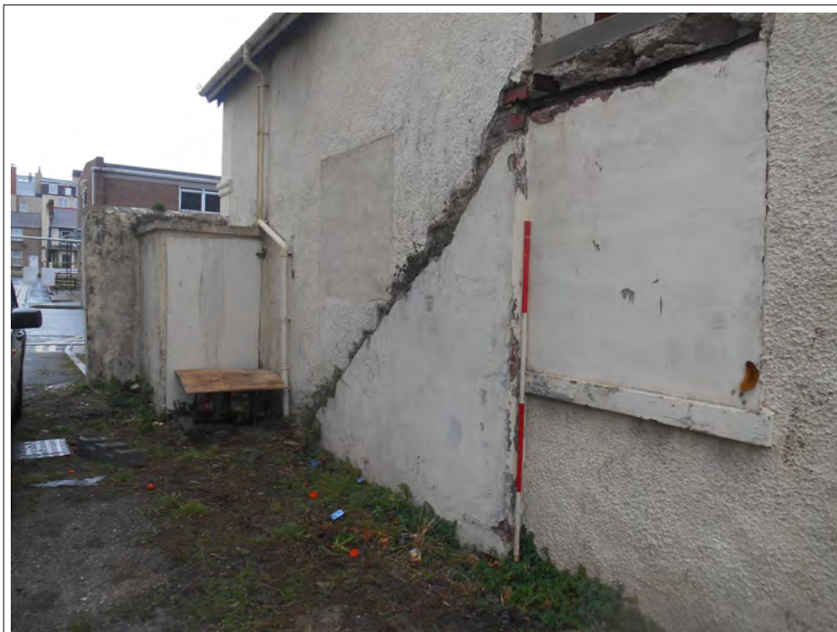
Plate 41. Outbuilding attached to garage behind facade wall. West facing wall. Scale 2m
