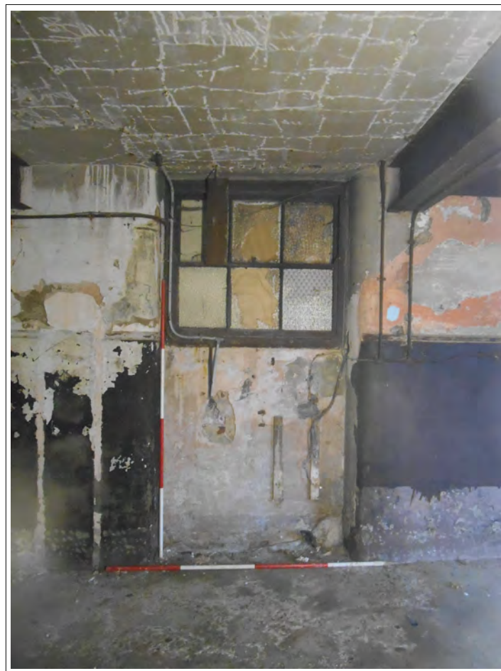
Plate 6. Remains of early door, subsequently transformed into a window which is currently blocked. Eastern facing interior wall. Scales 2 x 2m
