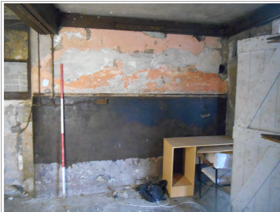
Plate 4. East facing wall of ground floor interior, with dado rail. Scale 2m
