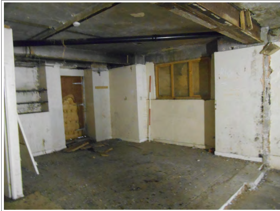
Plate 9. East facing wall. 1960's Window subsequently repaired. North facing wall with back entrance. Not original. Scale 2m
