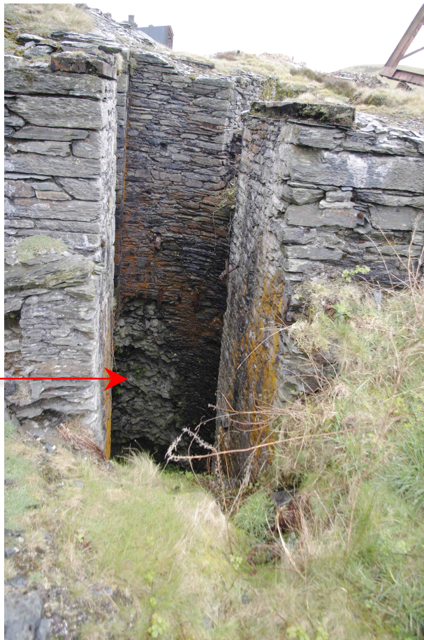
Photo No 4: The recent collapse in the shaft of the stone lining (lighter coloured rock) arrowed.
