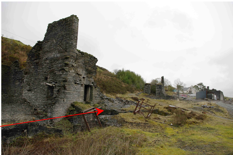
Photo No 2: View taken from edge of path of the Engine House and shaft
