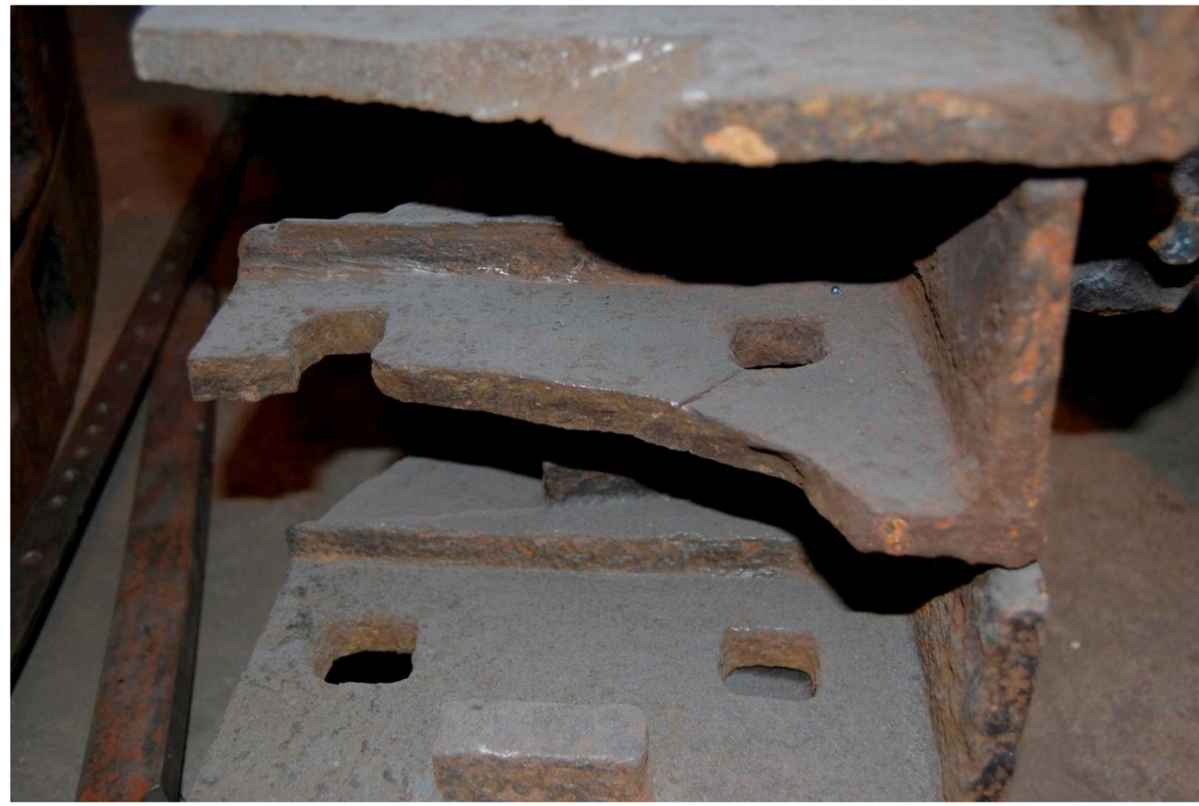
Fig 24 11/05/2010 Typical defects to Wheel Rim sections – fractures and loss of fabric where Spokes are connected to Wheel Rim segments. Repaired by splicing mild steel and welding.
