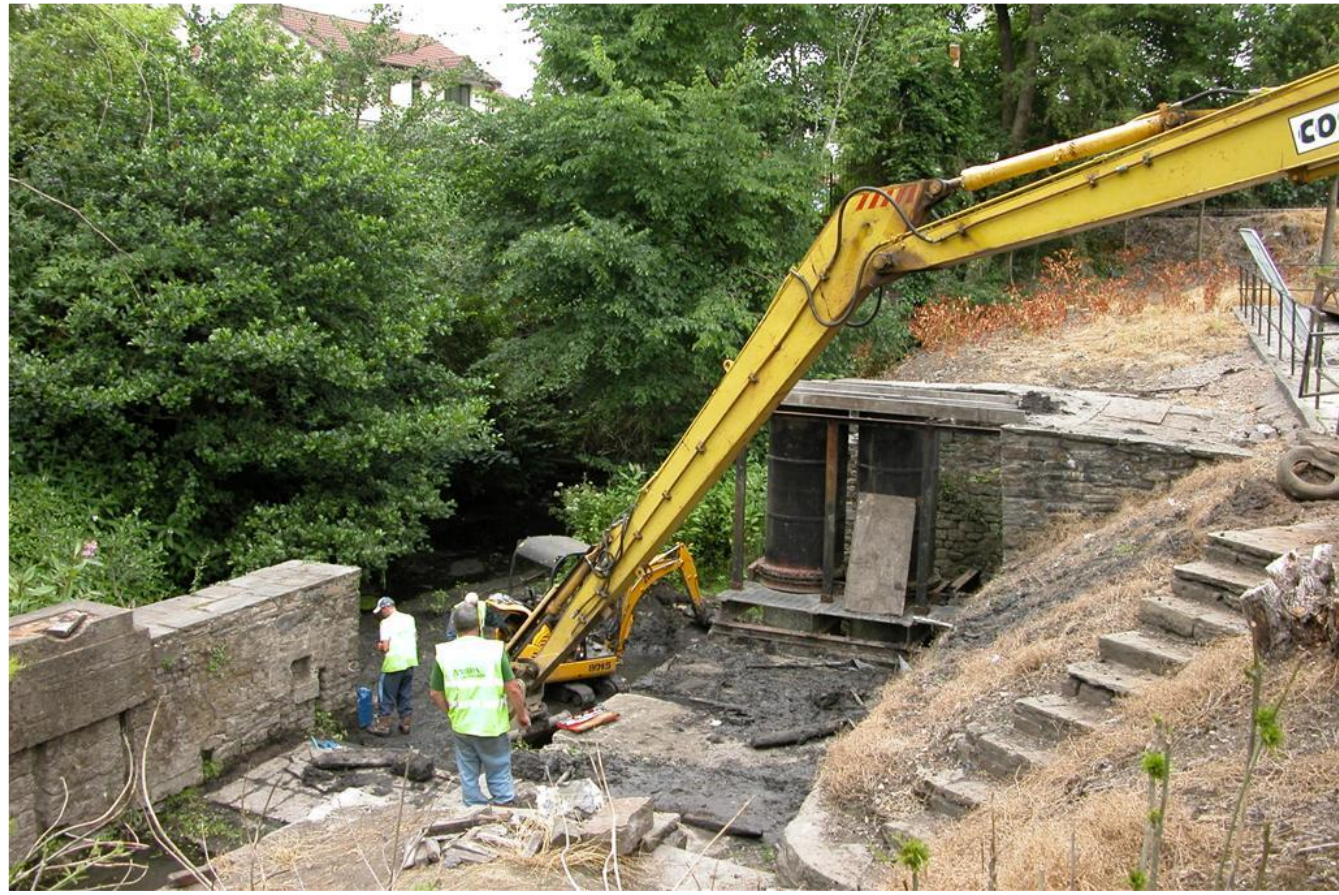
Fig 17 09/07/2010 Excavation of the Head-race and Wheel Pit. Large excavator plant used to lift material away, mini excavator used to collect debris.
