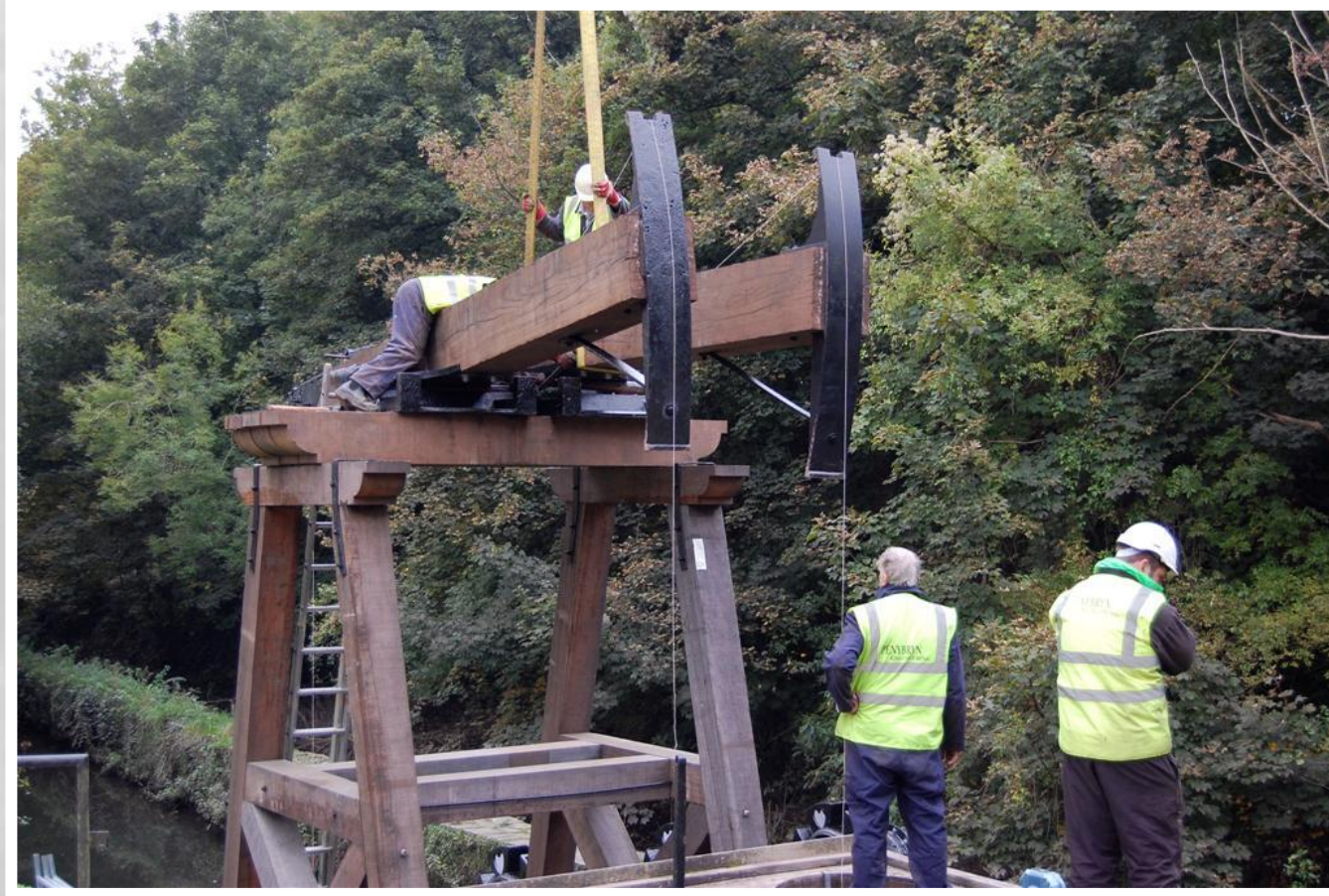
Fig 56 14/10/2010 Near-side Rocker Beam lowered into position on bearing saddle. Saddles adjusted to final alignment.
