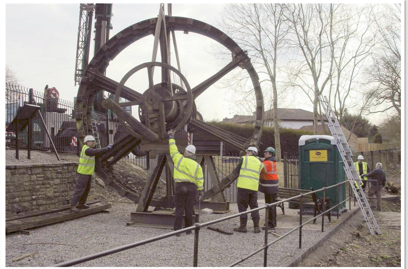
Fig 14 11/03/2010 Wheel rims, axle and crank arms lowered onto temporary jig to allow dismantling by hand.
