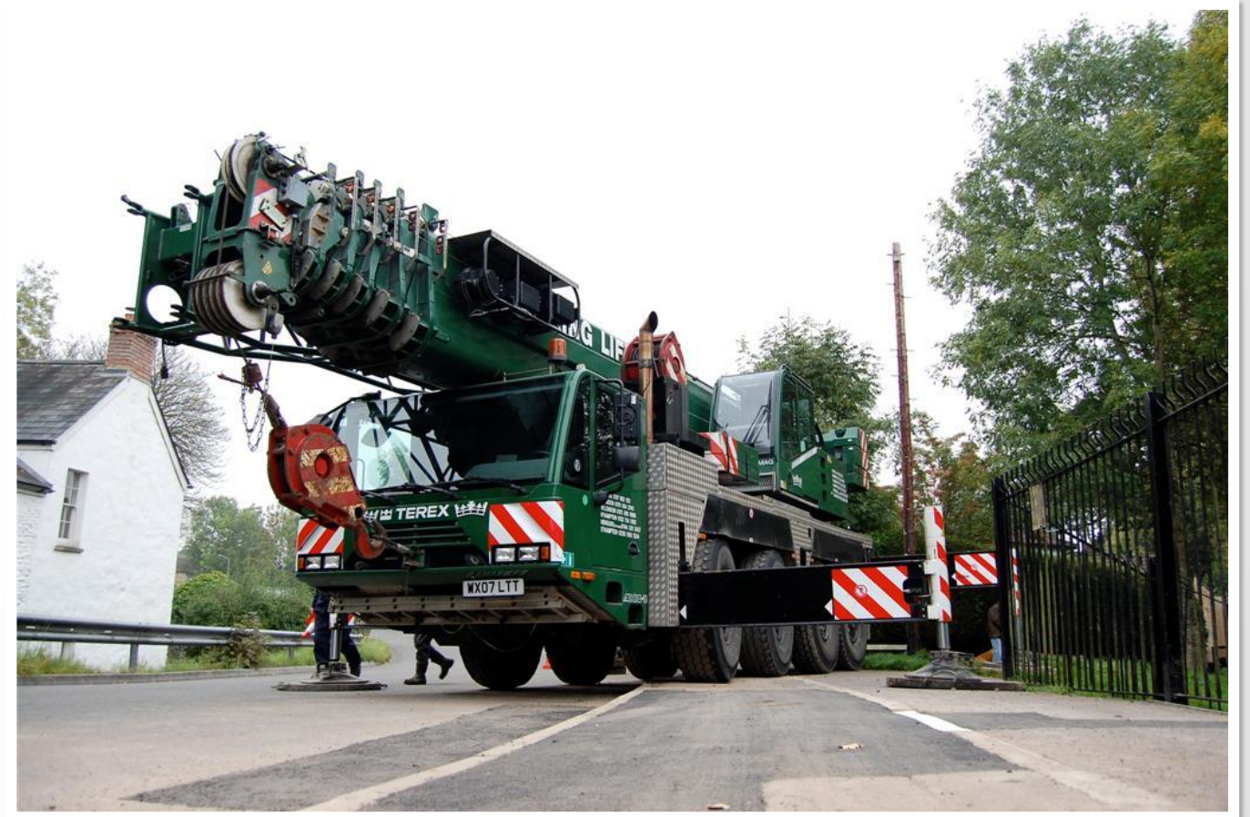
Fig 43 14/10/2010 Crane in position on Ty Mawr Road in preparation for main lifting operation.
