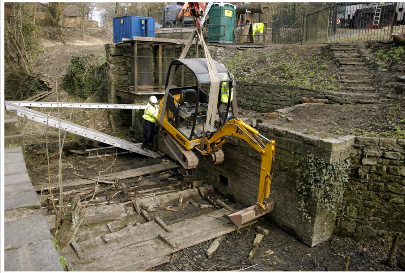
Fig 15 11/03/2010 Mini excavator lowered into wheel pit to assist with removal of silt and accumulated debris. Note Pump cylinders remain in-situ.
