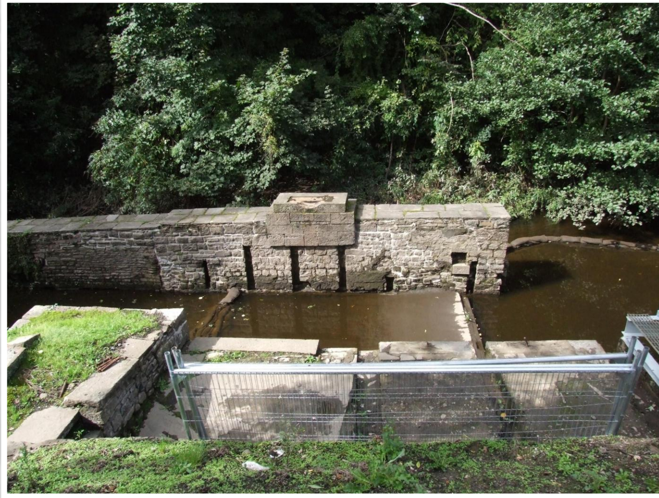
Fig 19 15/09/2010 View on Island wall following masonry conservation work to repair defective areas of original mortar pointing etc.
