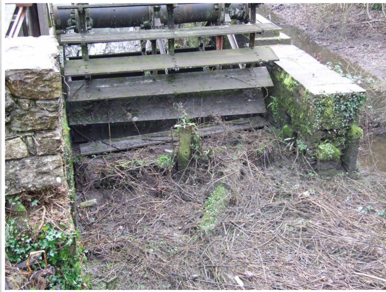
Fig 3 14/01/2009 View of the Wheel pit as viewed from the Head-race. Note significant accumulated silt, debris and vegetation. Remains of original sluice gate frame visible.
