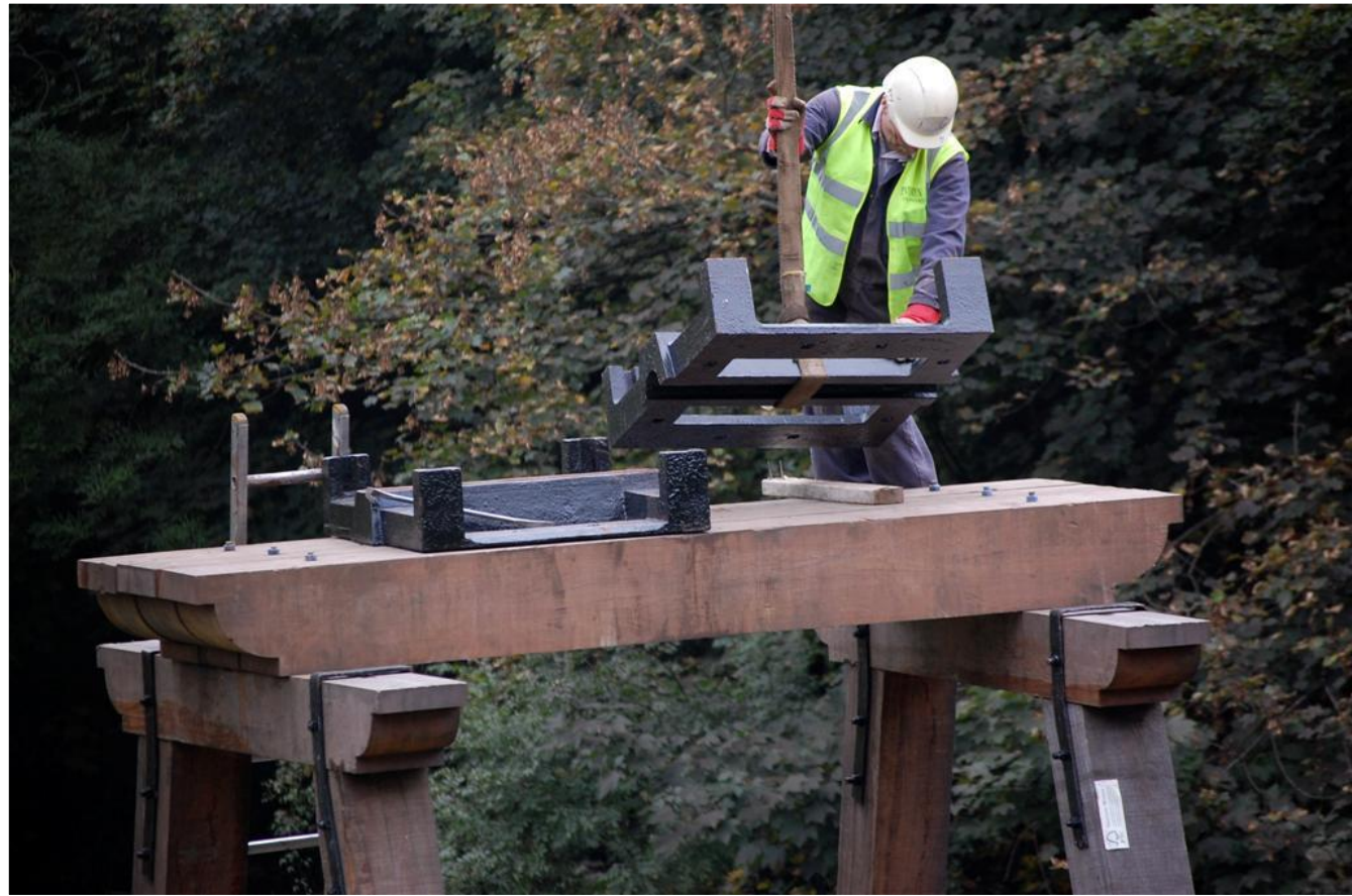
Fig 54 14/10/2010 Rocker Beam bearing saddles lowered into position atop the A-frame. Final alignment to follow once Beams are in place.
