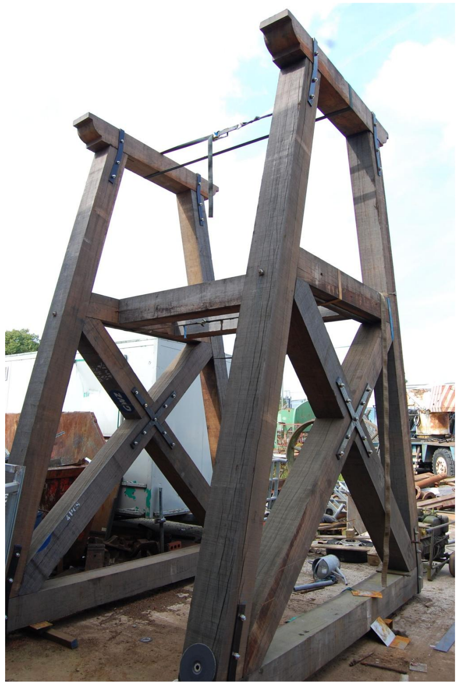
Fig 40 03/09/2010 Assembly of replacement A-frame in Ekki hardwood. Original metal braces reused and decorated.
