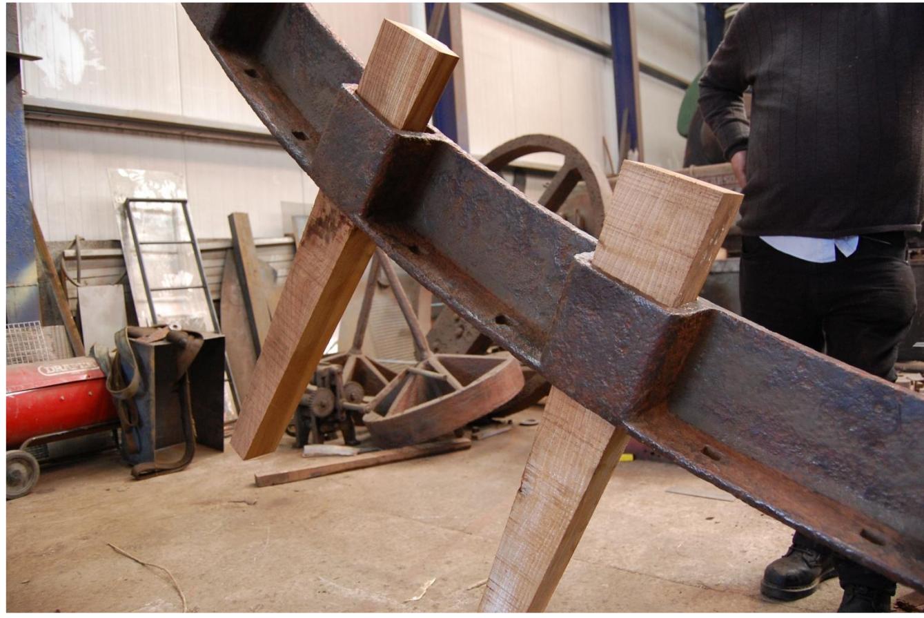
Fig 36 03/09/2010 Replacement Paddle Blade Brackets in Elm to match original details. Original Brackets were all defective, lost or rotten.
