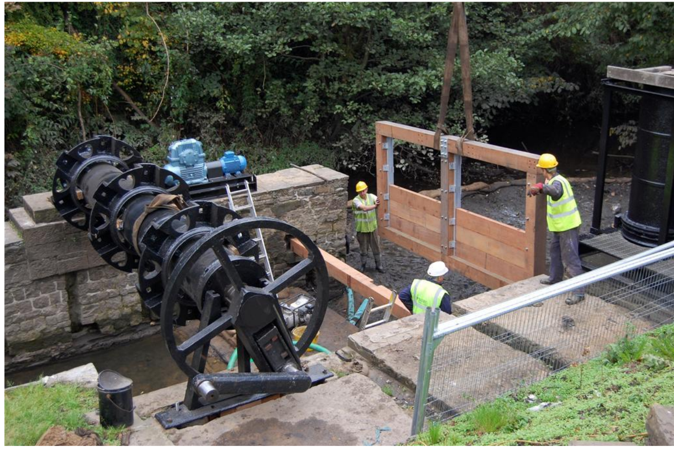
Fig 50 14/10/2010 New Sluice Gate frame lowered into position across Head-race. Cross-beam into original beam pockets already in place.
