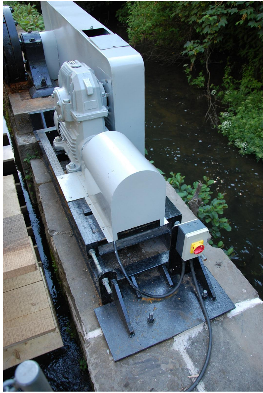
Fig 70 02/06/2011 View of completed motor frame showing position of Cintec anchors to bedrock (below isolator switch). Safety cover to chain drive shown.
