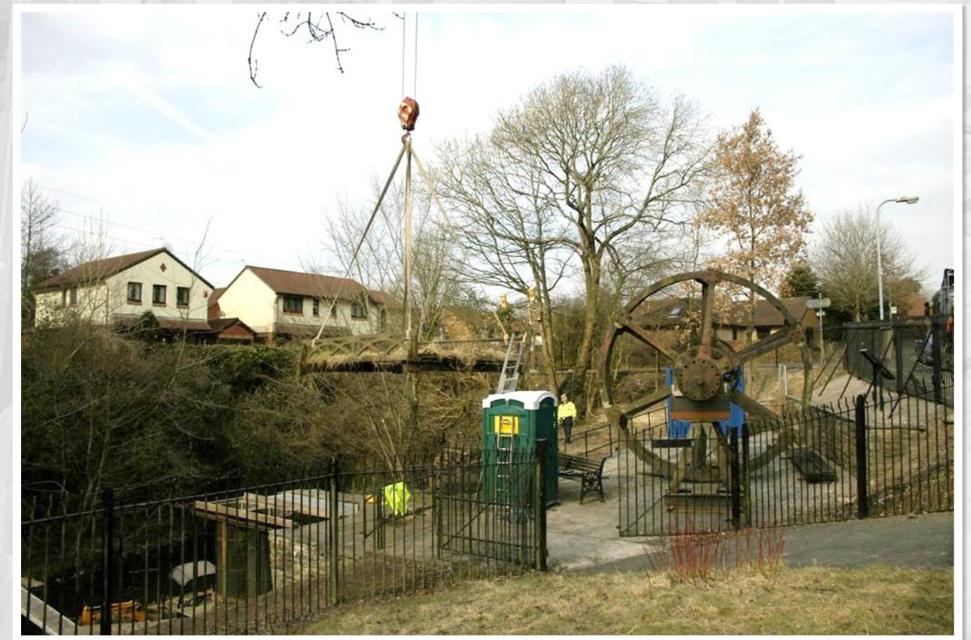
Fig 16 11/03/2010 Original Tow-path Bridge lifted from area of wasteland into the site enclosure for safe storage and display.
