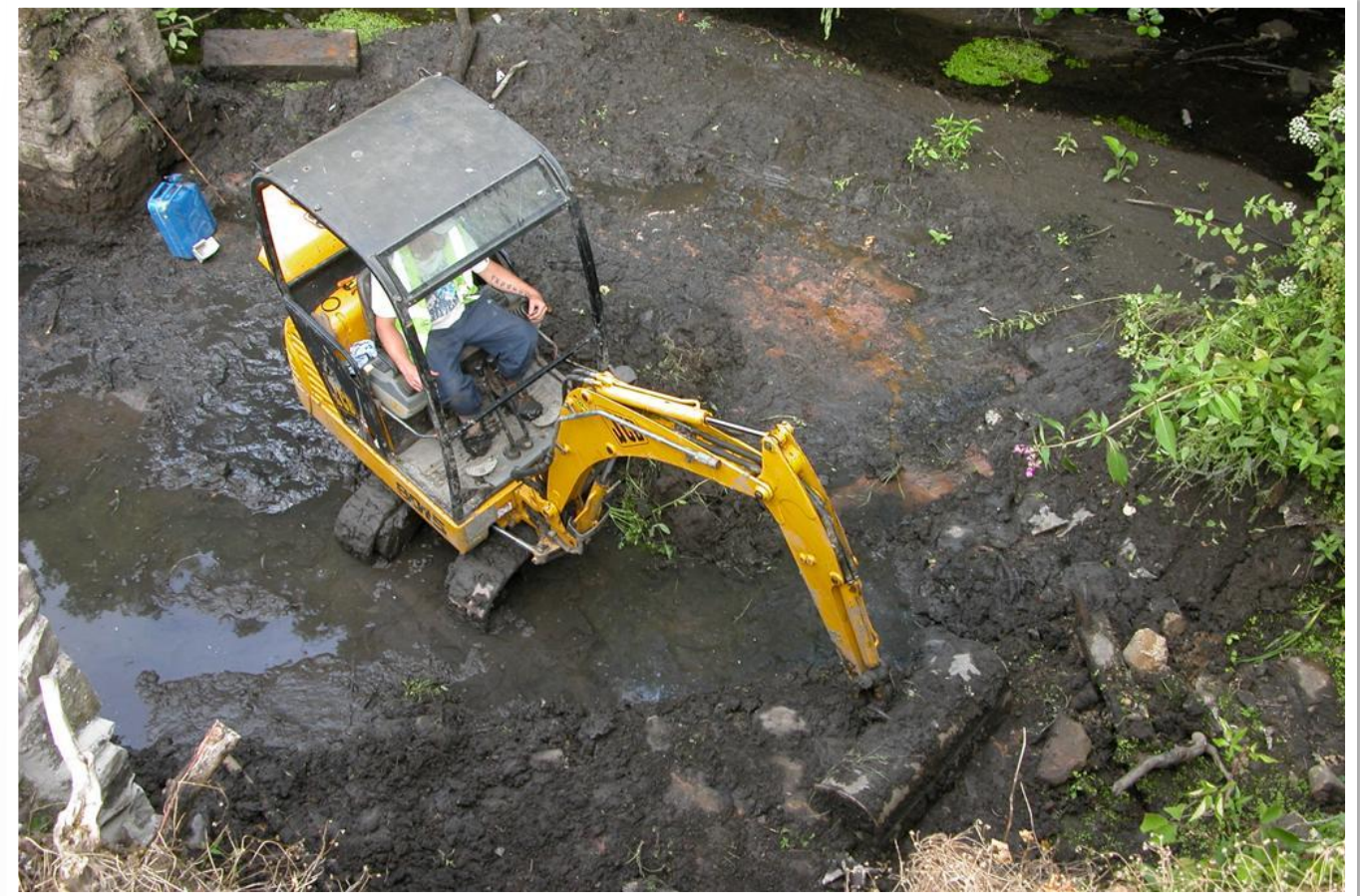
Fig 18 09/07/2010 Mini excavator collecting silt and debris from the Head-race. Bedrock exposed close to the final surface levels. Investigation could not establish the position of original Filter Screens.
