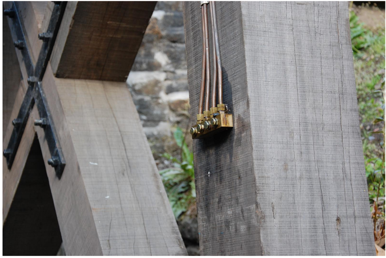
Fig 62 02/07/2011 Lubrication access points mounted on A-frame for safe lubrication of Rocker Beam bearings saddles.
