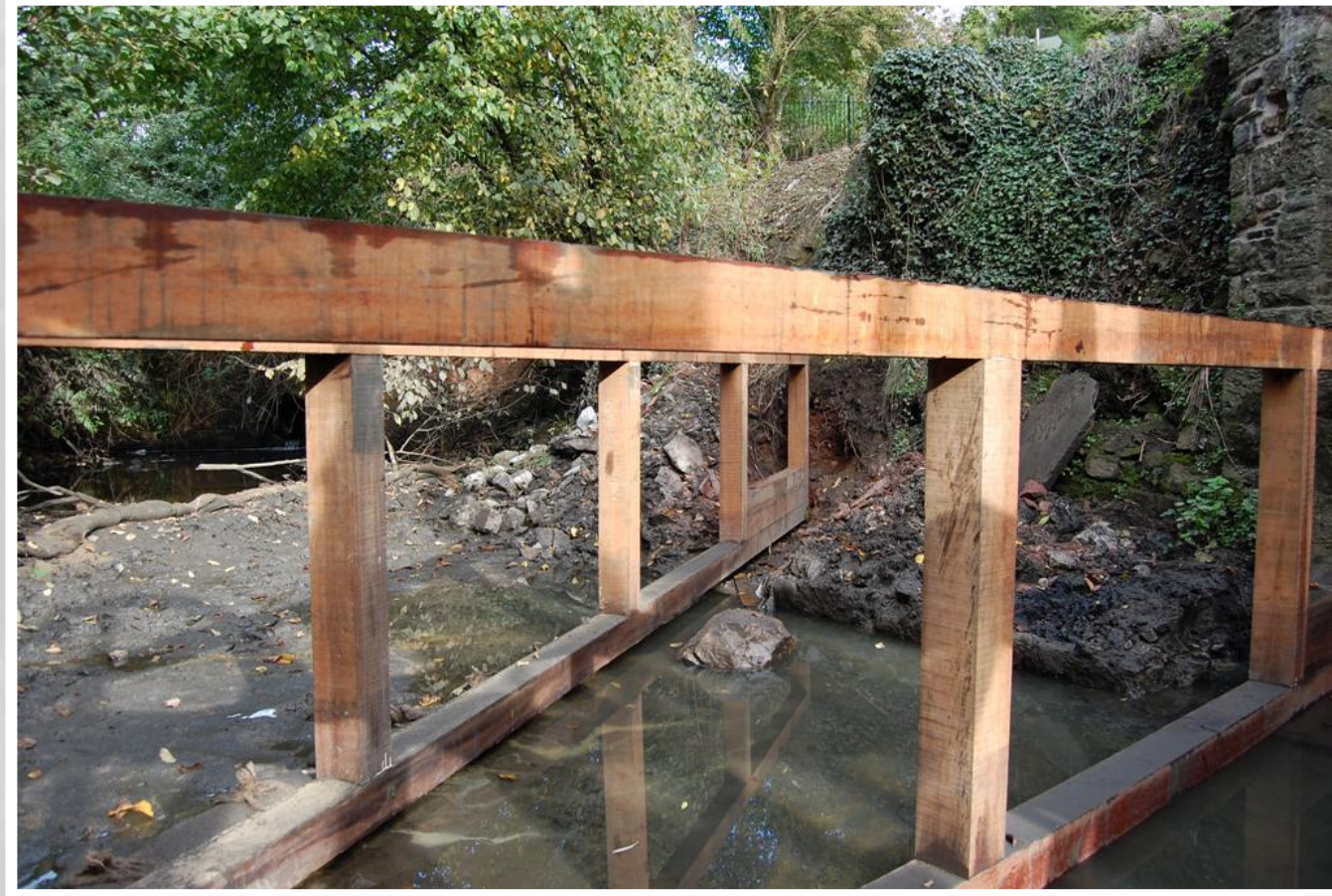
Fig 64 21/10/2010 View from the Wheel Pit showing alignment of Filter Screens. Infill bar and mesh not fitted.
