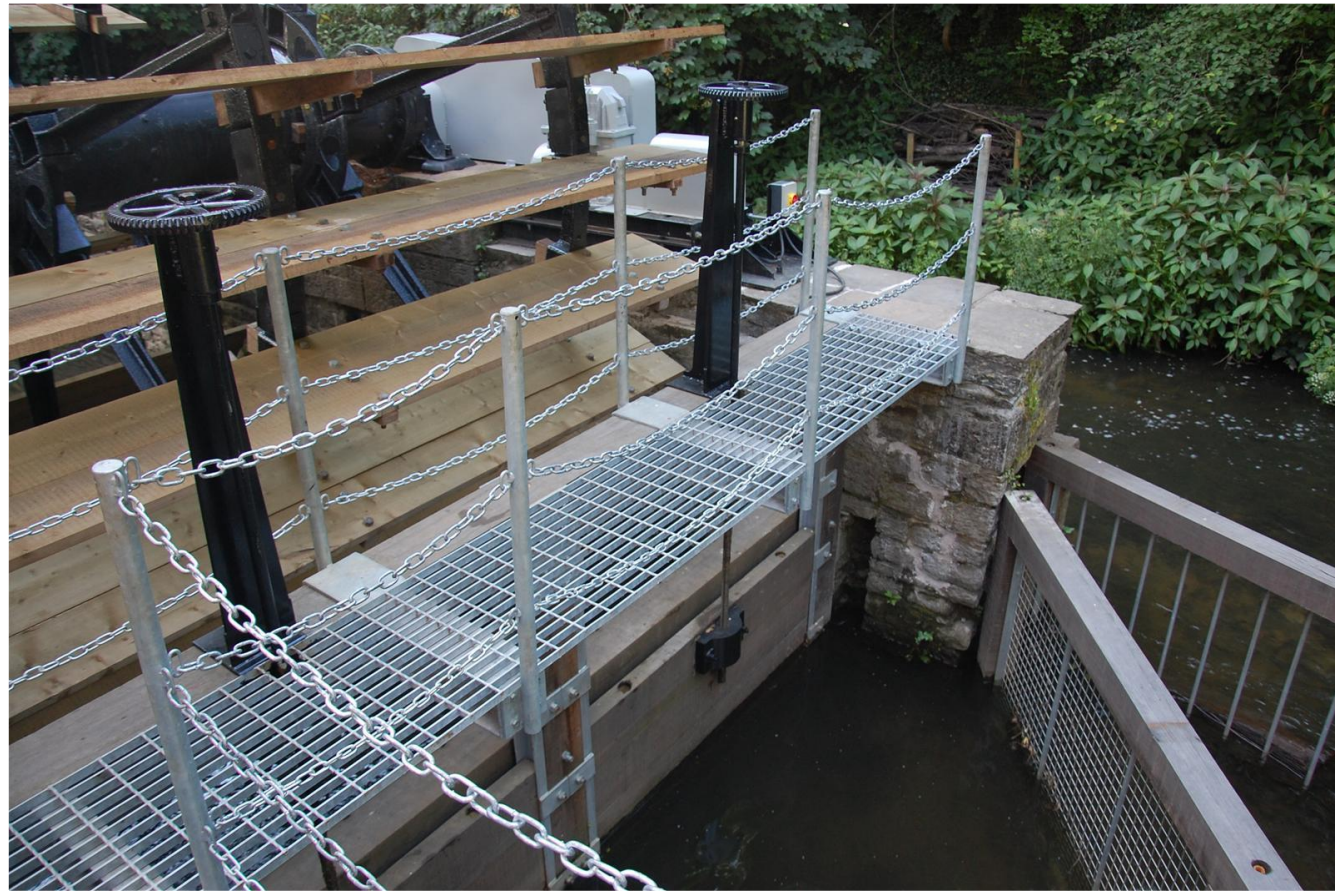
Fig 66 02/06/2011 View showing new galvanised mild steel access walkway fixed to replacement Sluice Gate frame. Sluice Gate lifting mechanism also shown, one for each Gate.
