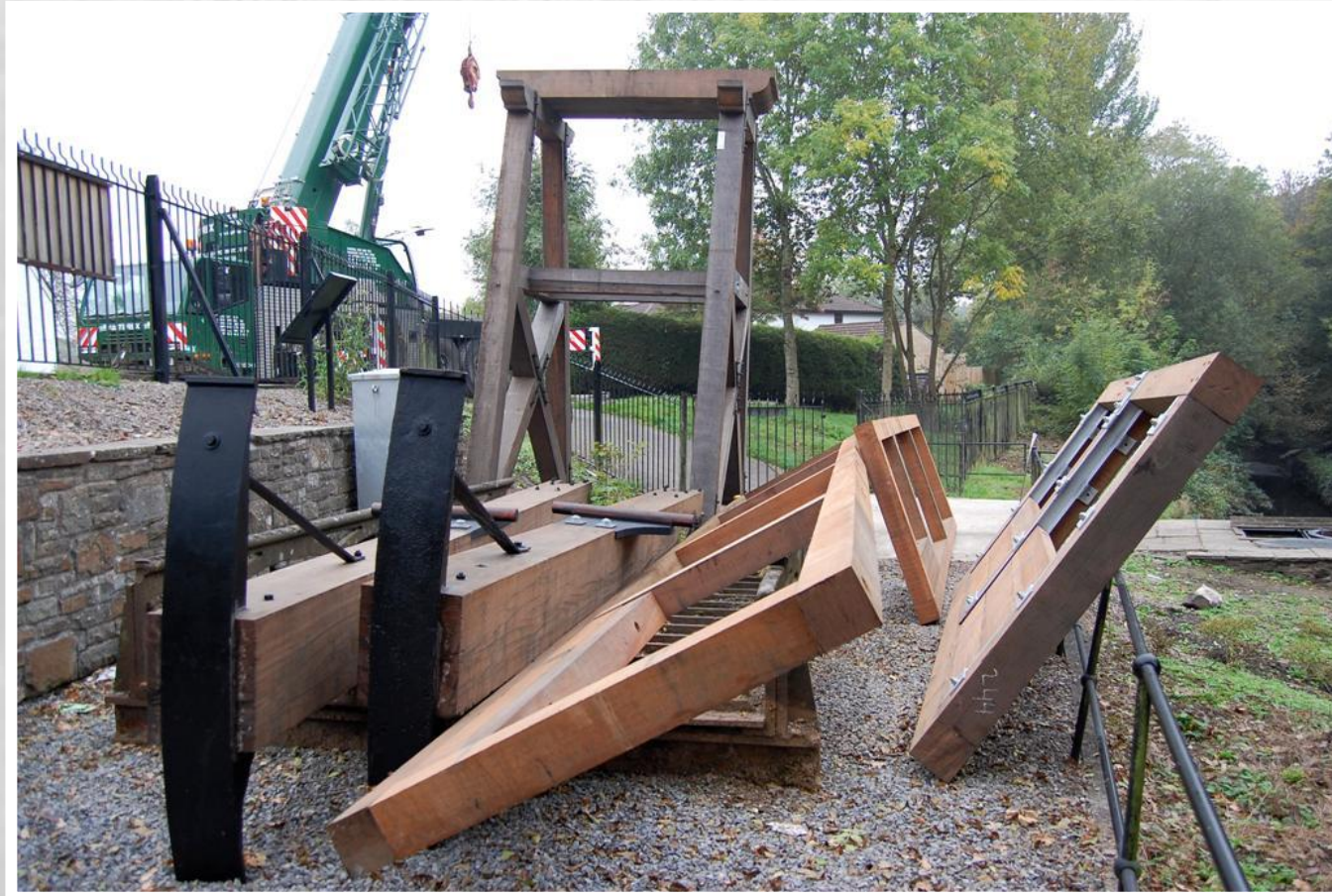
Fig 44 14/10/2010 Replacement Rocker Beams and associated metalwork, Sluice Gate and Filter Screen frames delivered to temporary location on site.
