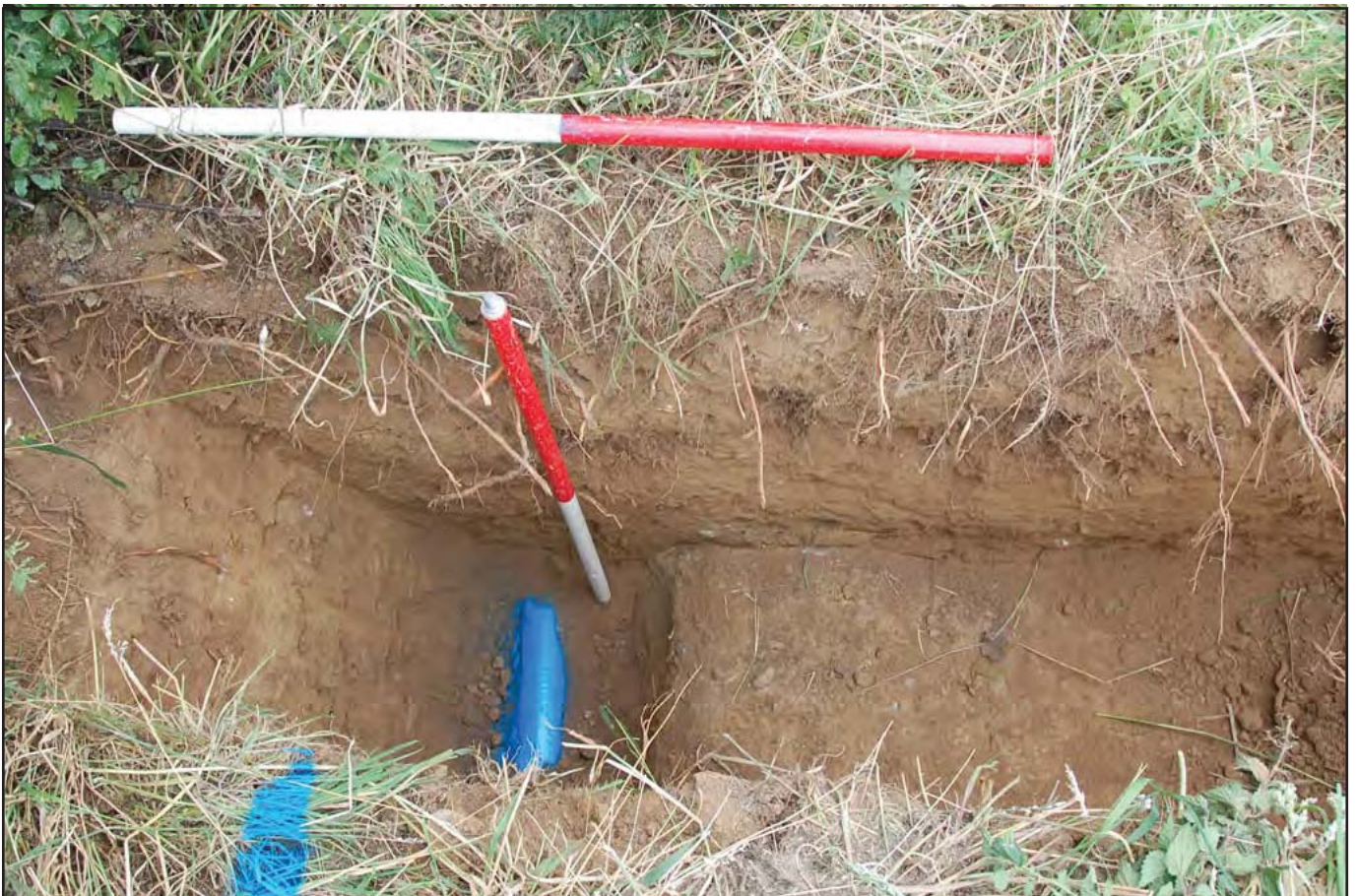
Plate 08 - East facing section of TH13 showing the bpainted water main and natural surface to the right.
