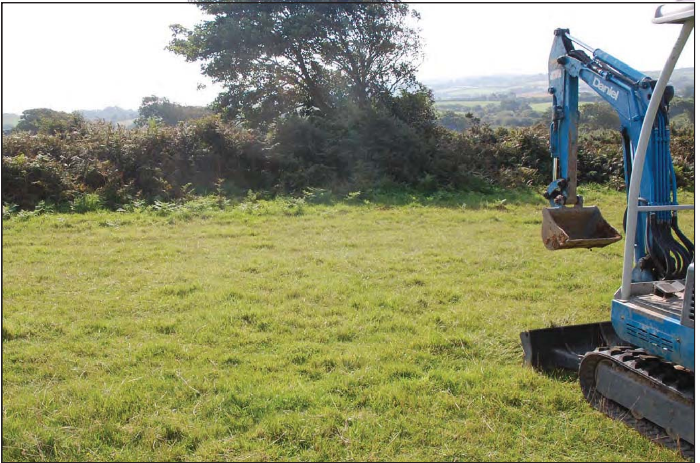
Plate 011 - Location of TH15 with the Abersoch to Llanengan road the other side of the tree.
