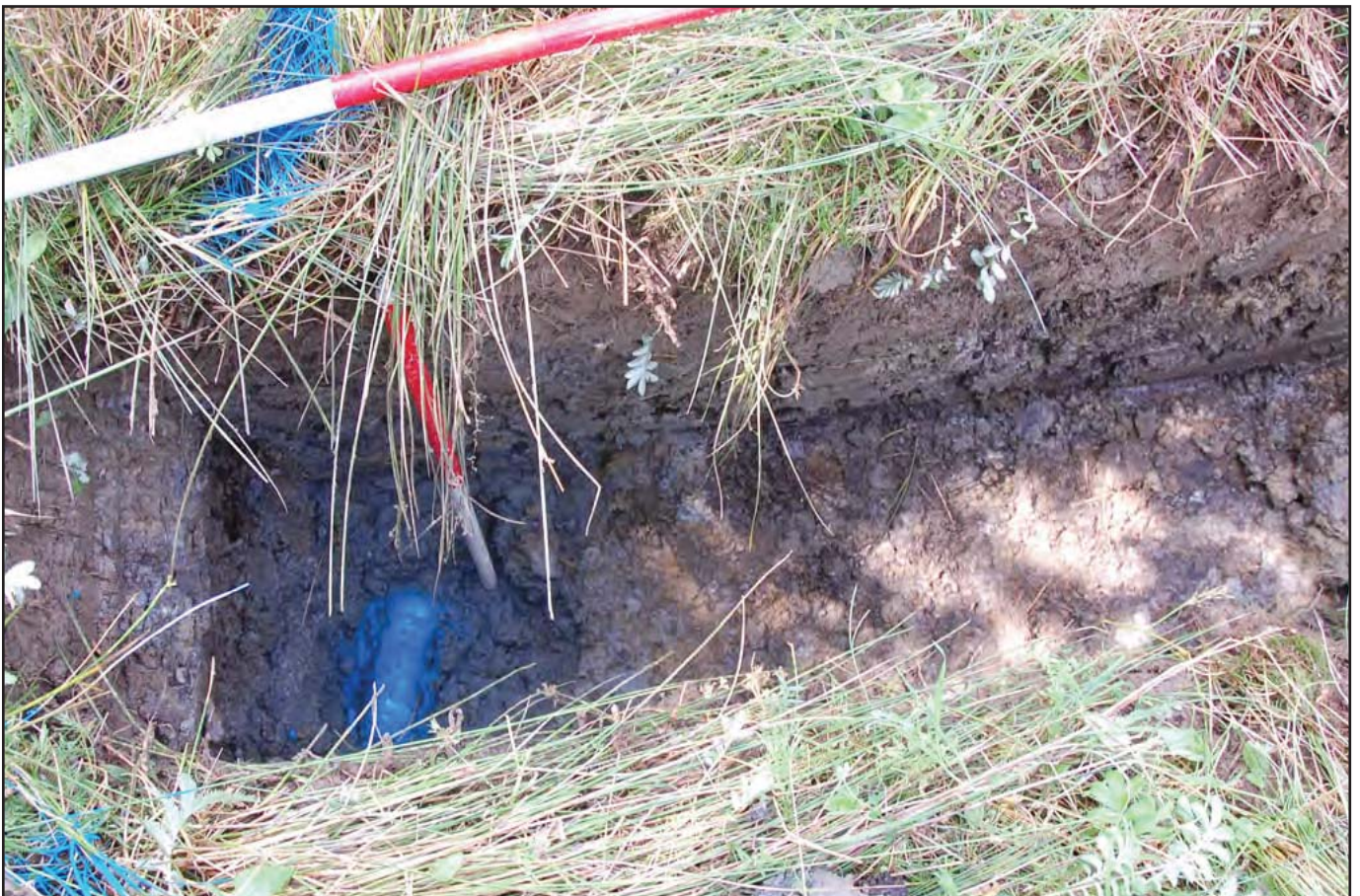
Plate 02 - Excavated test hole showing the water main (blue paint) cut into thye natural.
