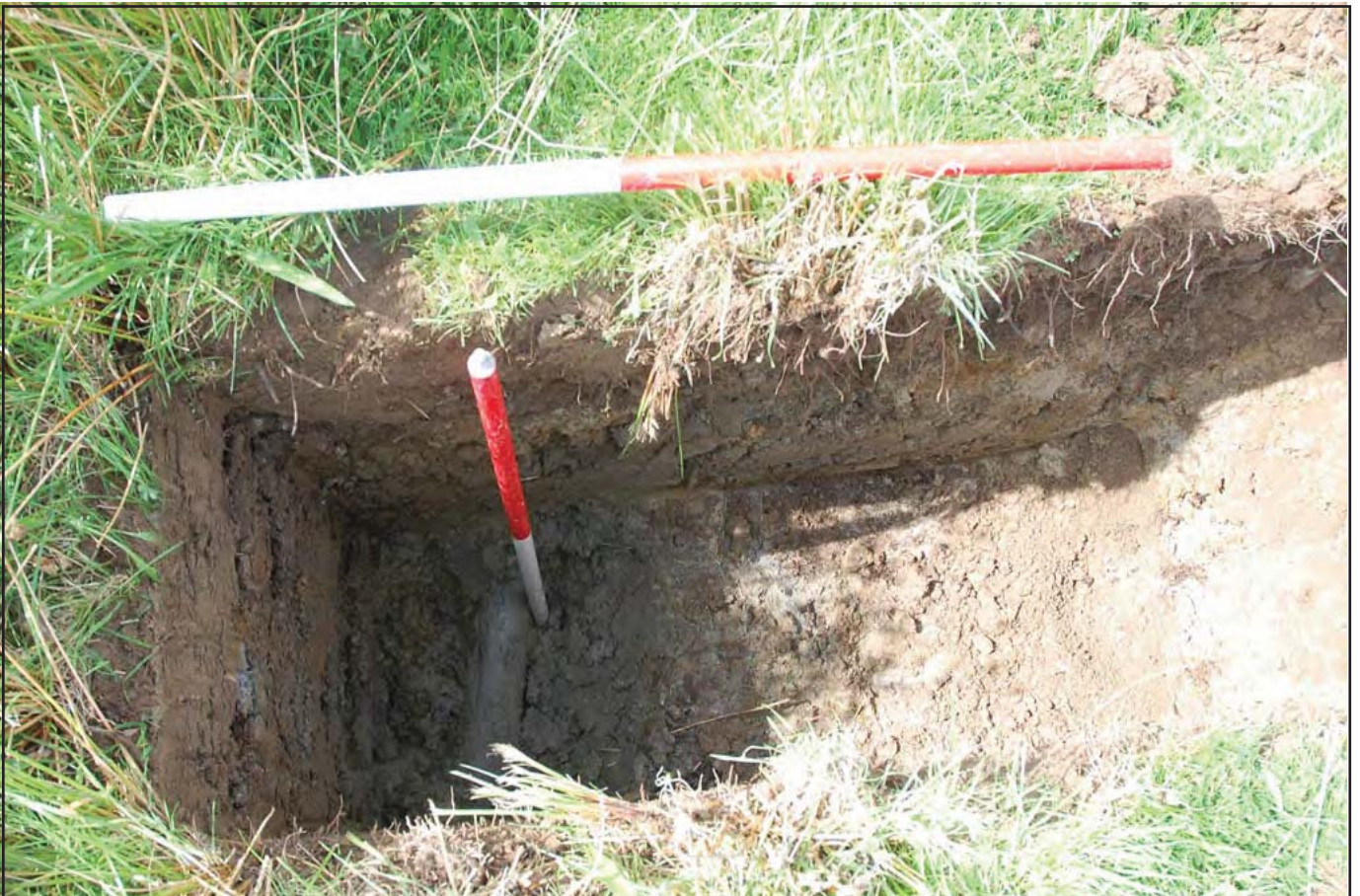
Plate 04 - Post excavated section of TH11 with the water main next to the ranging pole.
