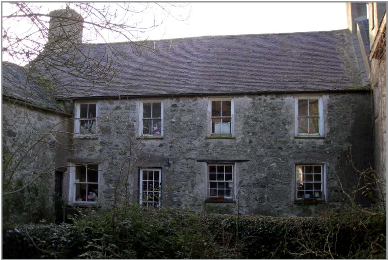
Plate 9: Gronant north facing elevation showing building B with four sash windows on the first floor, two 12-pane windows to the east and a four pane to the west. The change in masonry shows that the window east of the door was once a door
