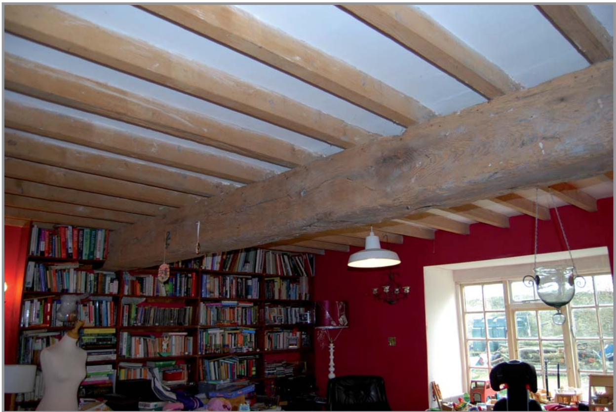
Plate 14: Gronant building B living room facing south west showing the large square axial beam which runs east to west across the entire of building B
