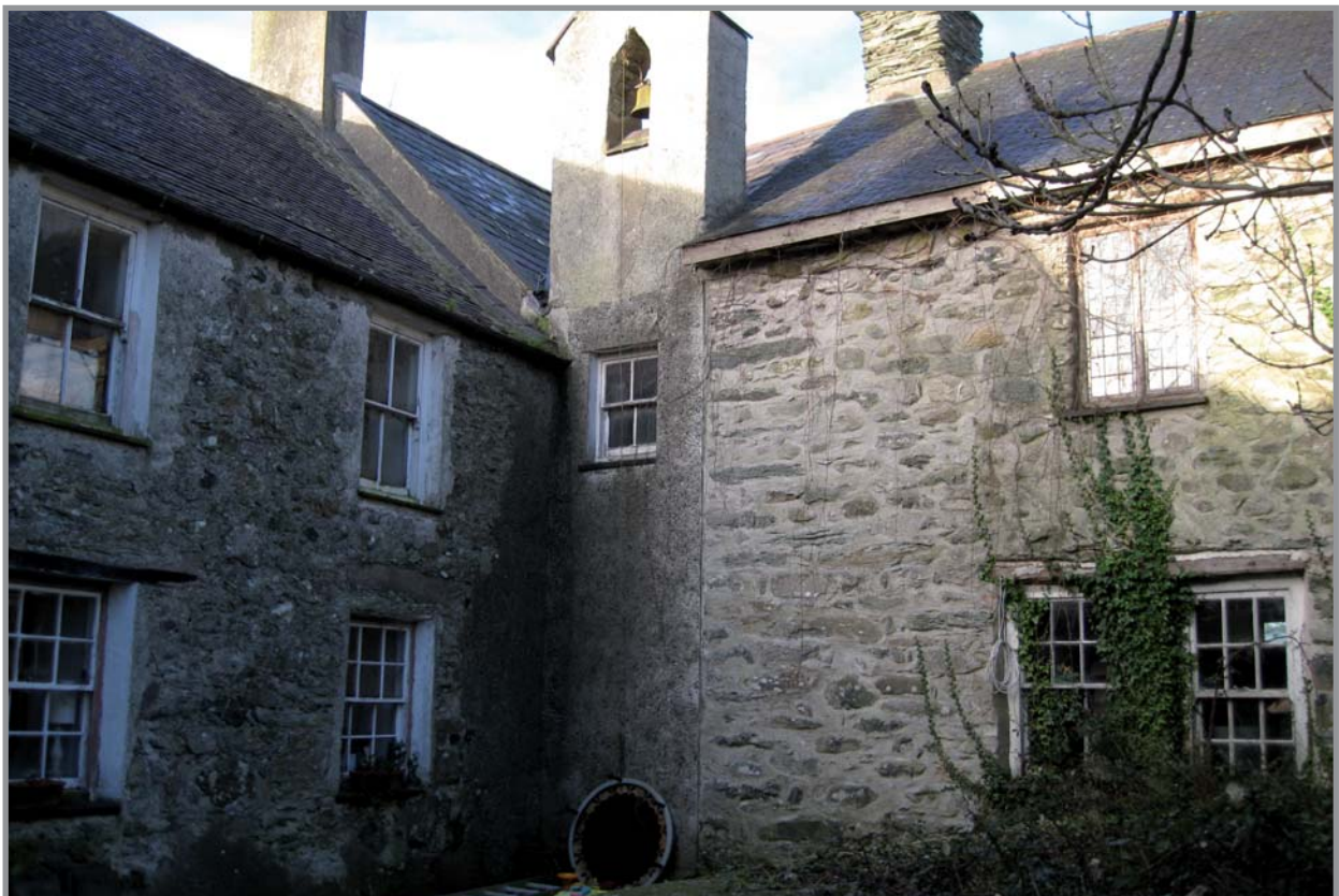
Plate 10: Gronant facing north-east showing building A and B and the 19th century connecting wing bell tower with a small four pane sash window
