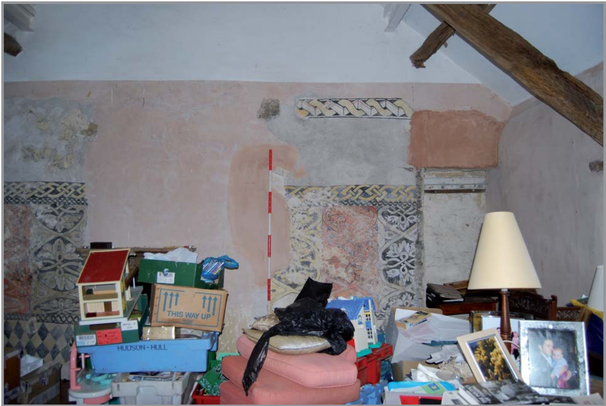
Plate 25: Gronant building A., first floor. Wall paintings discovered and restored in c. 1986. Facing south.
