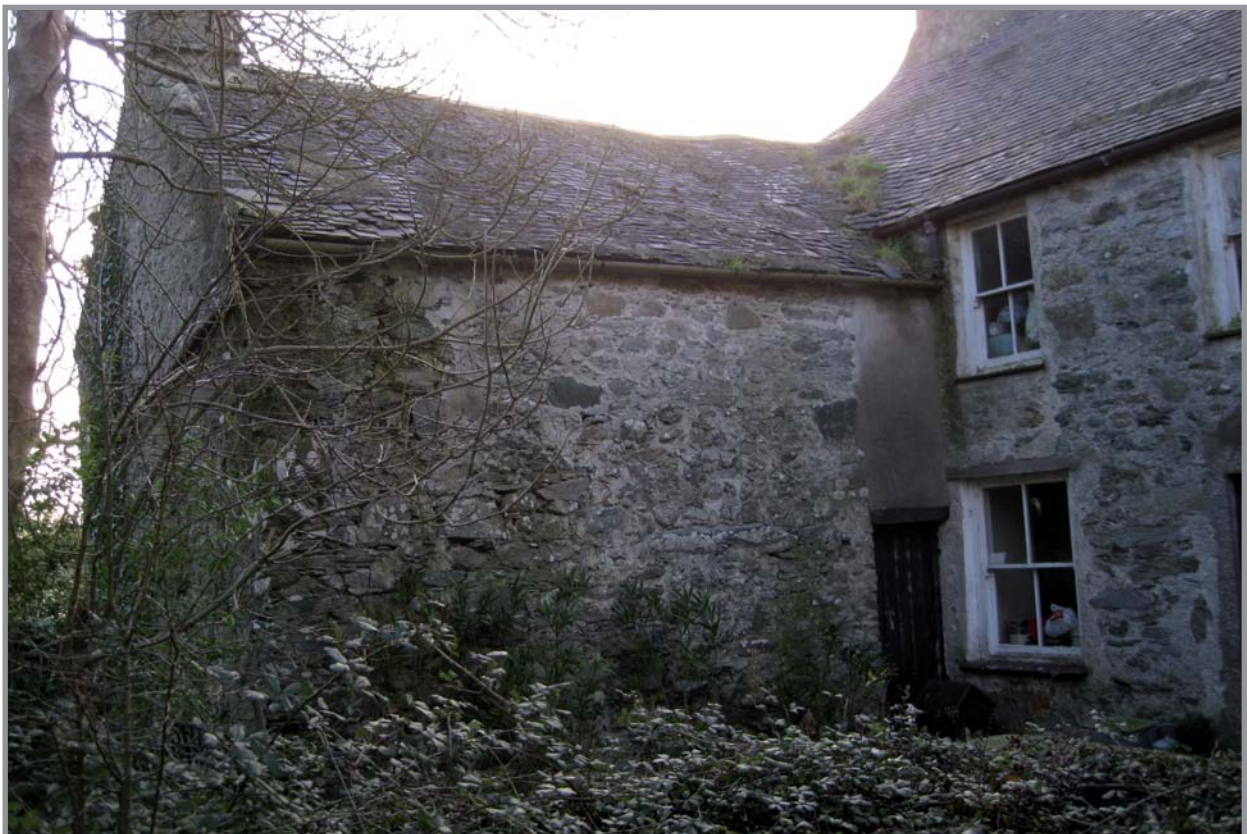
Plate 8: Gronant west facing elevation of building B and the attached 2 storey building
