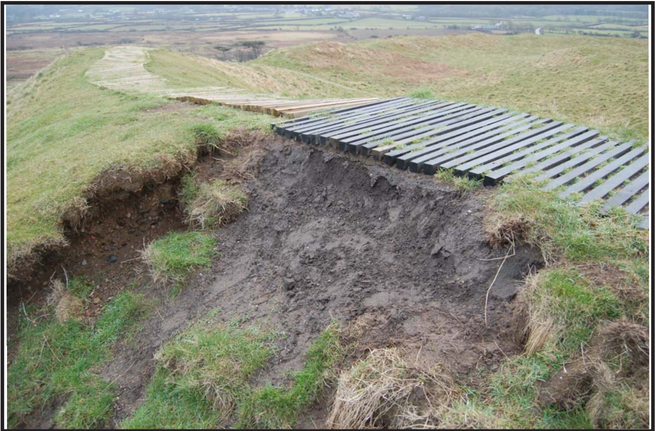
Plate 5 Redeponed soil, consolidation material brought in to stabilize and protect ramparts prior to laying pathway
