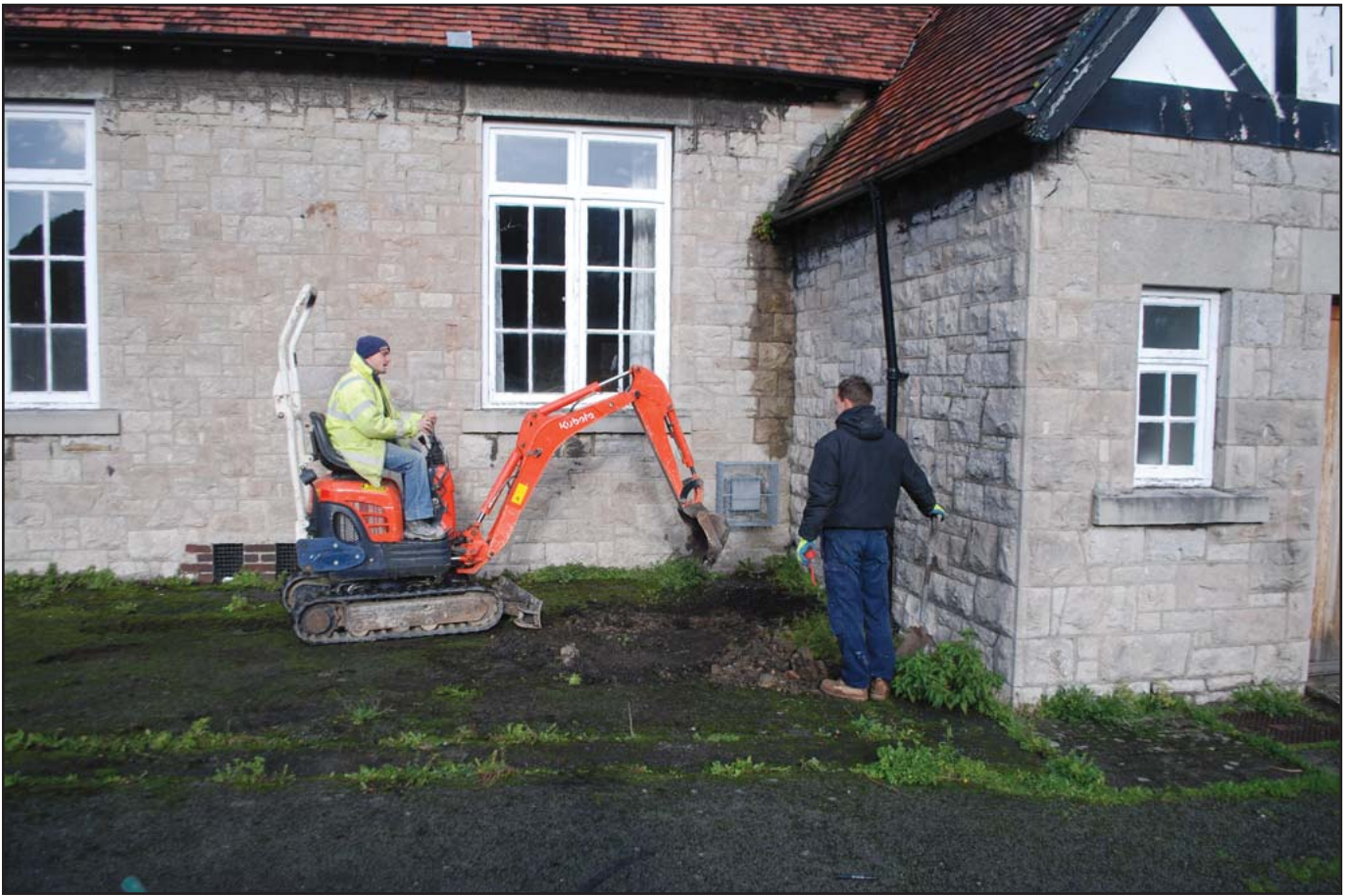
Plate 9: Church hall during initial ground works - View from Rose Hill Street to the South
