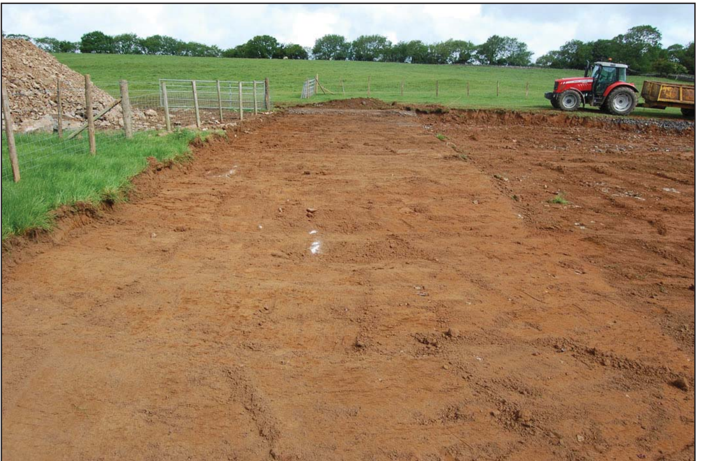
Plate 8: Post-excitation shot of the south-west end of the site, which was topsoil-stripped only.
