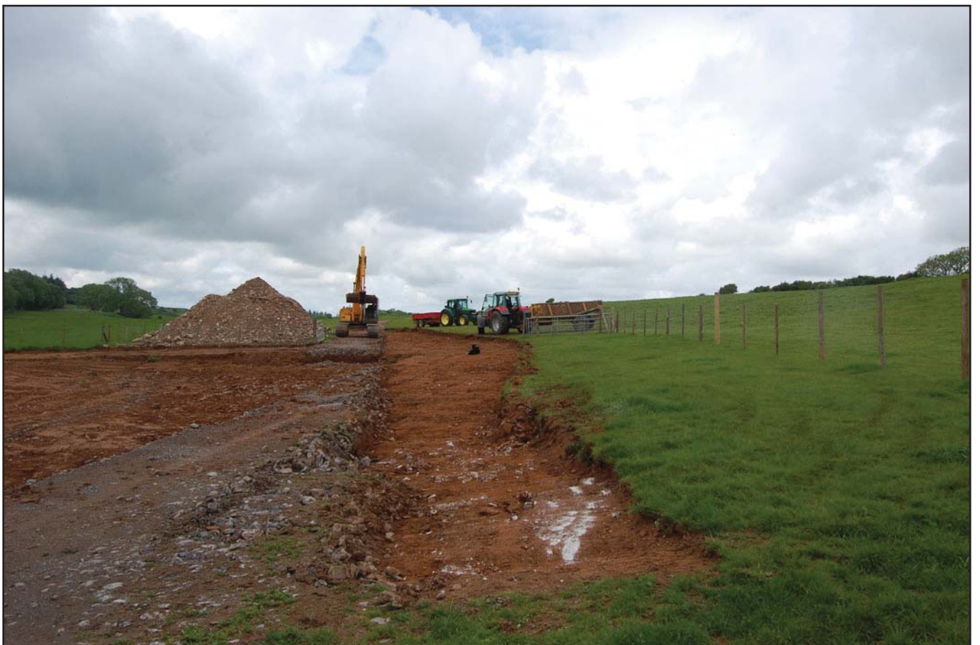
Plate 10: Post-excavation shot of the foundation trench for the replacement track (view from the north-east).
