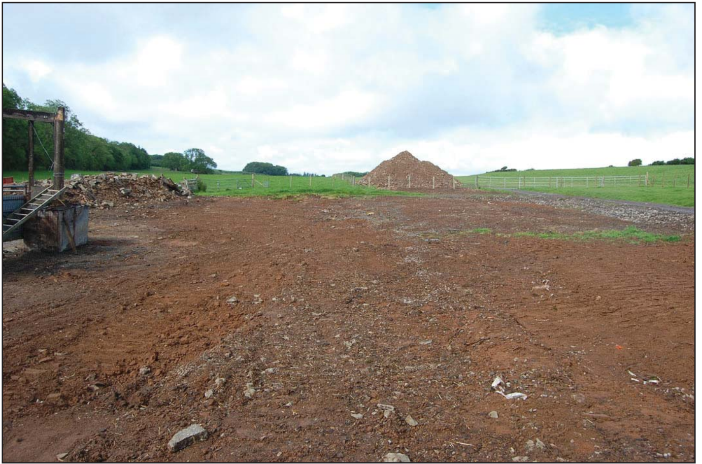
Plate 1: Pre-excitation shot of the site following the removal of the previous structure (view from the north-east).
