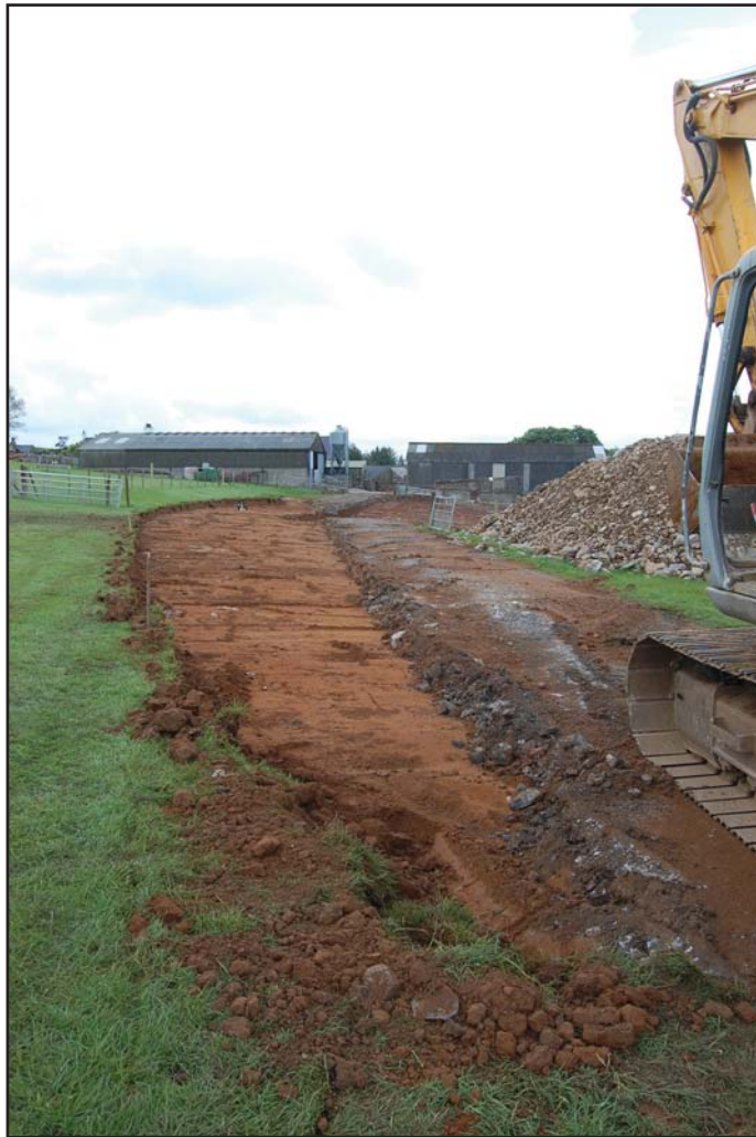
Plate 9: Post-excavation shot of the foundation trench for the replacement track (view from the south-west).
