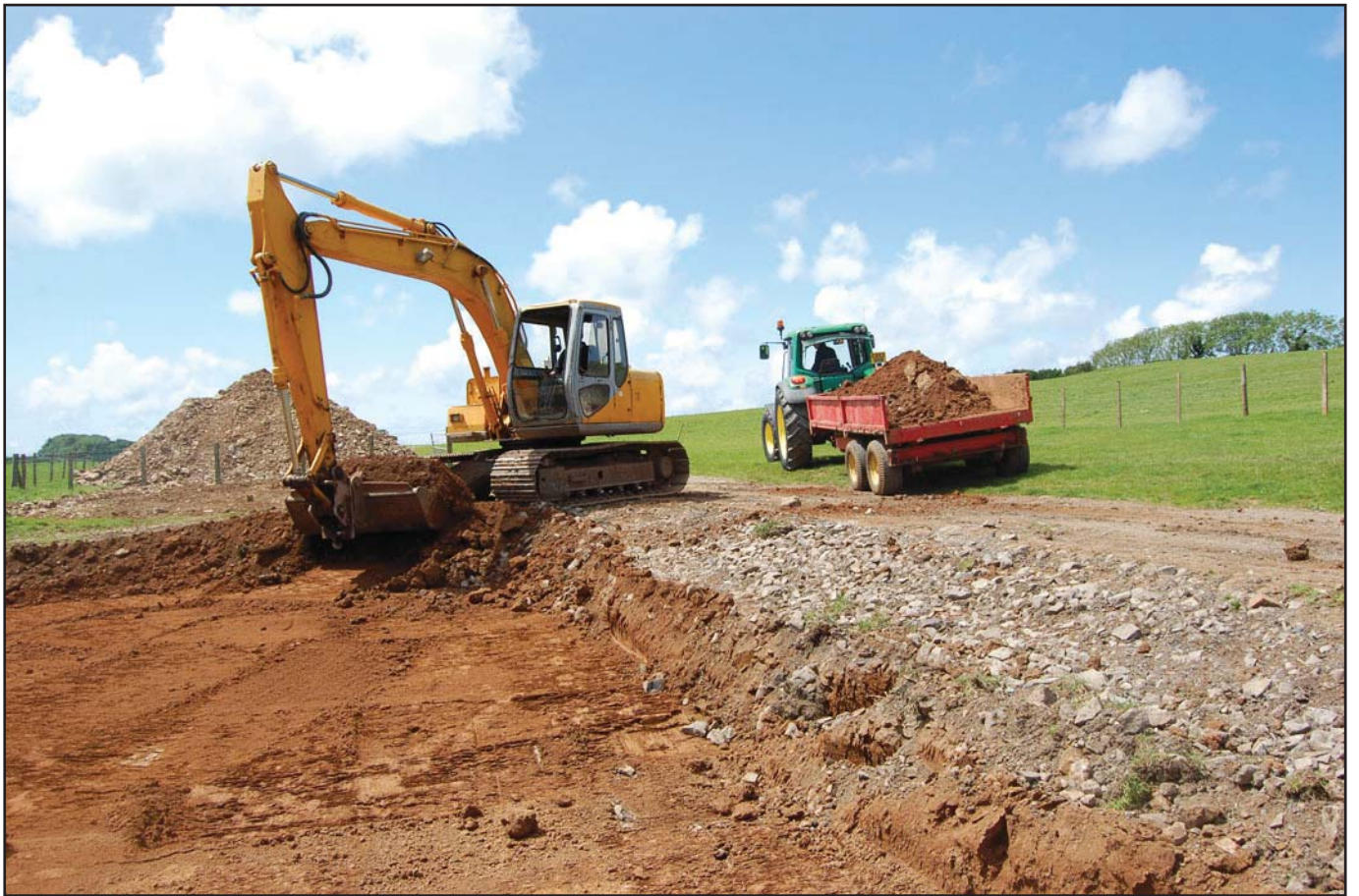
Plate 3: Working shot, showing excavation into the hillside along the north-western side of the plot.
