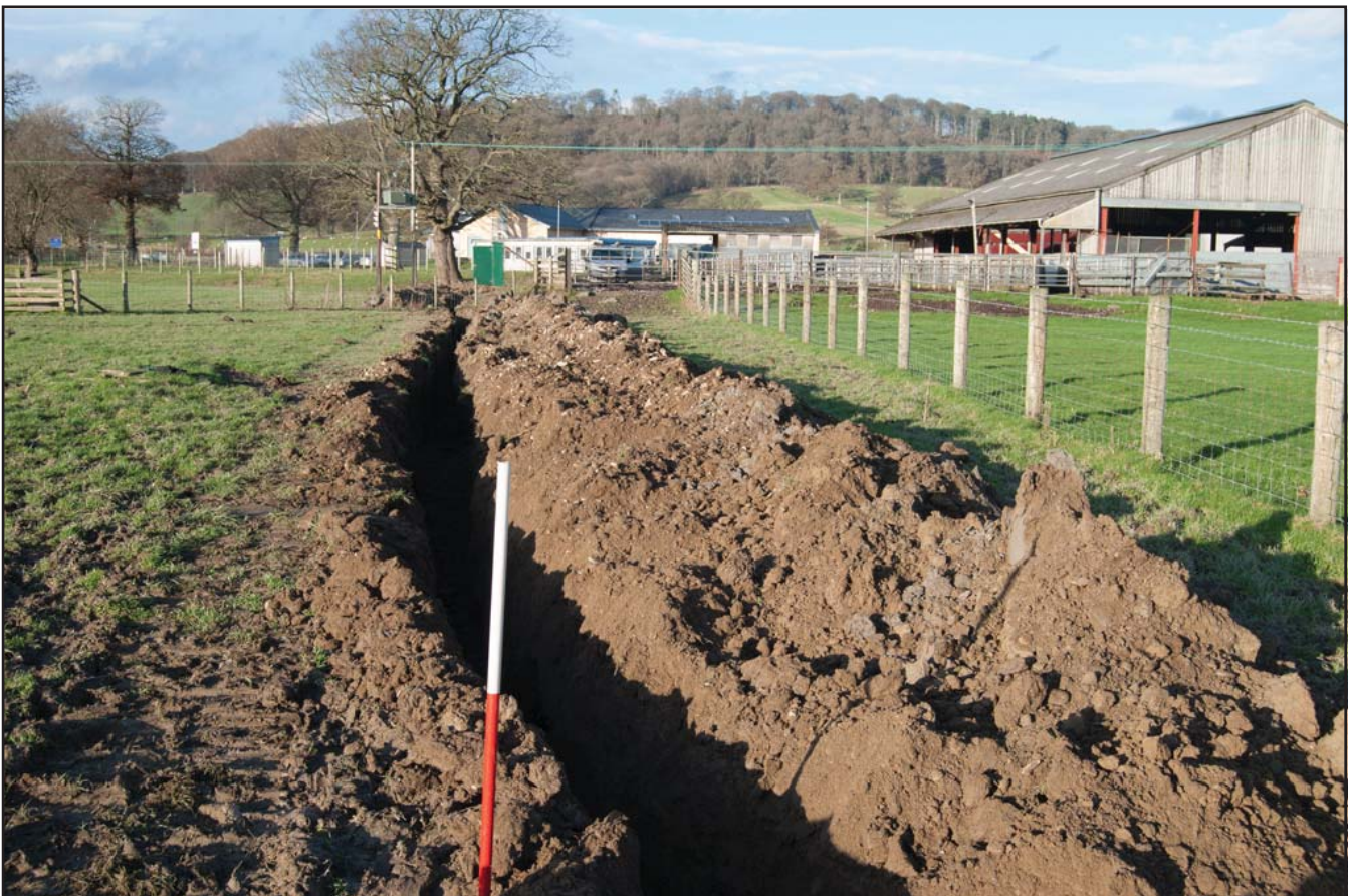
Plate 04: Trench by second transformer (west side of site) after excavation. View from south;1x1m scale.
