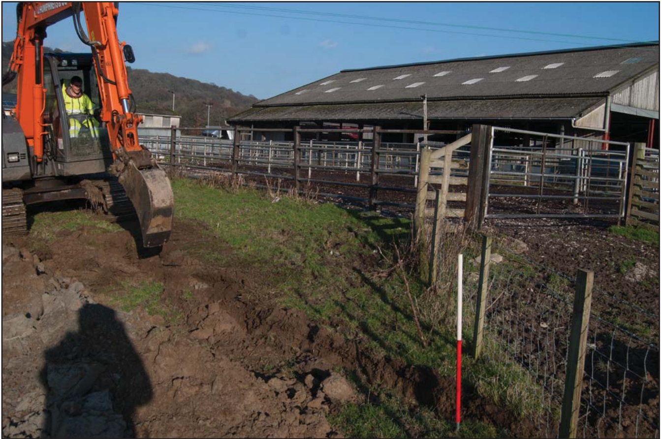
Plate 01: Working shot of trench by the second transformer (west side of site) during excavation. View from south; 1x1m scale.
