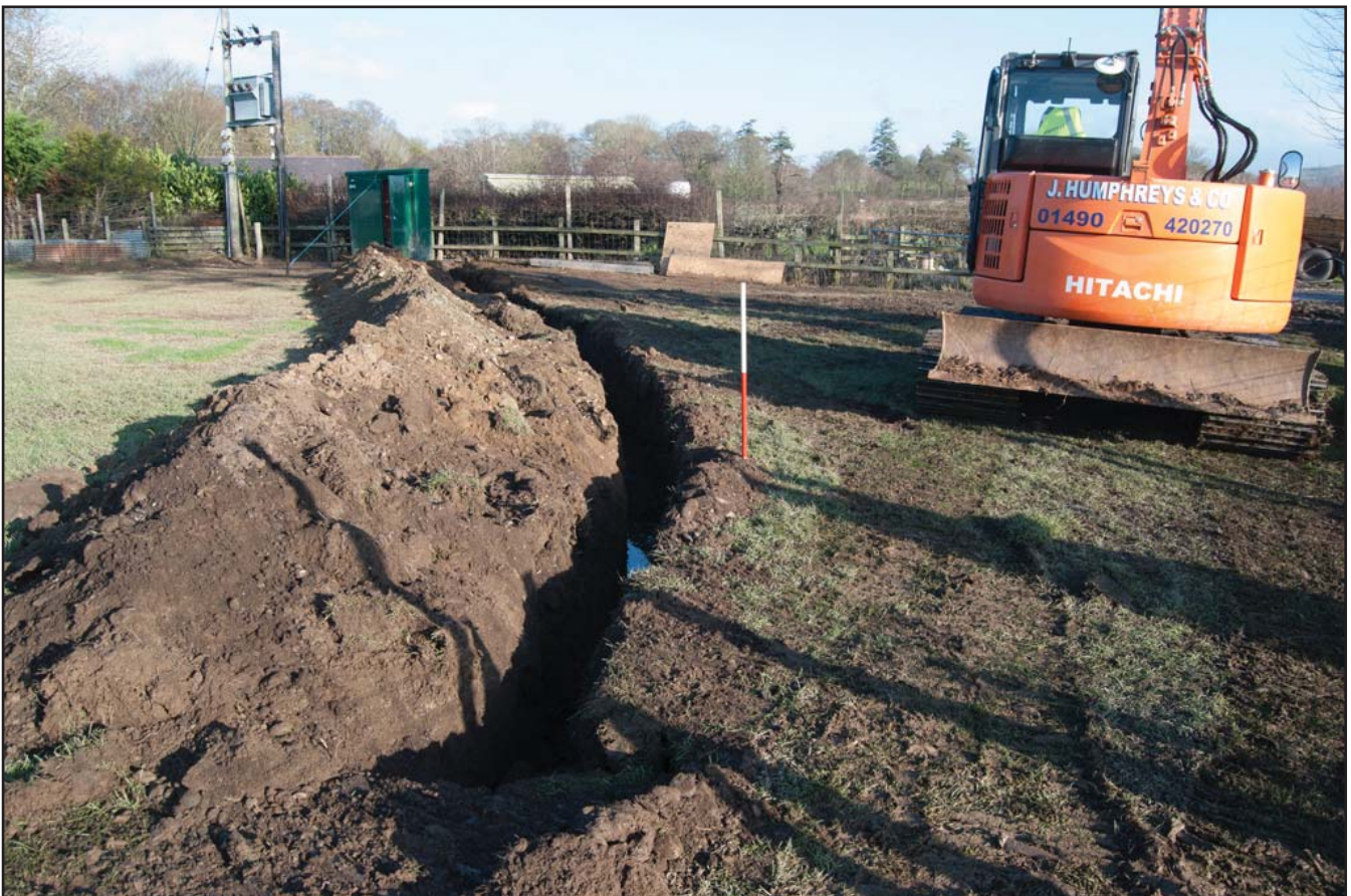
Plate 02: Excavated trench by the first transformer (east side of site). View from west; 1x1m scale.
