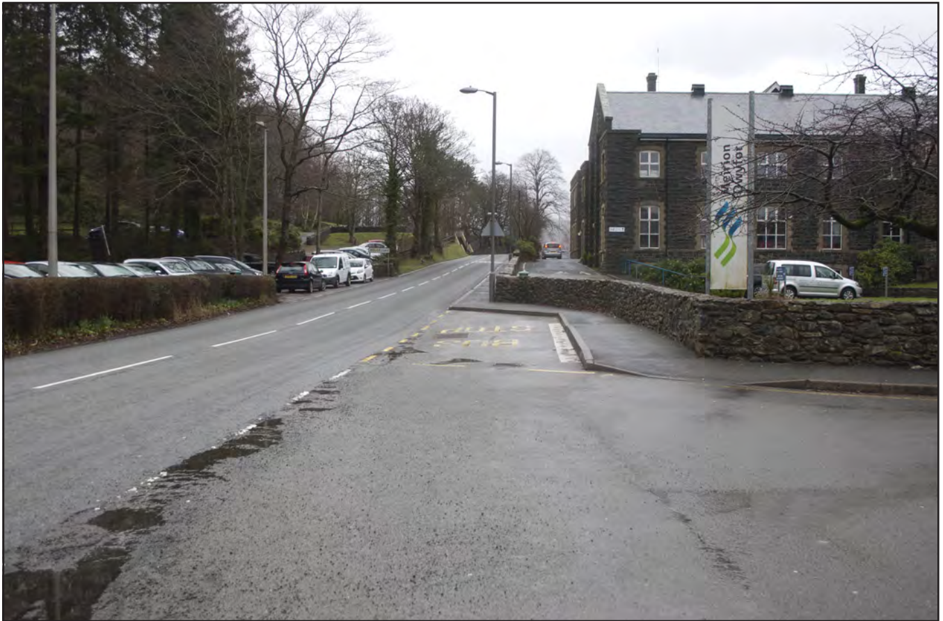
Plate 20: Section G-H: View west along street at Colrg Meirion Dwyfor, with pipeline route under pavement
