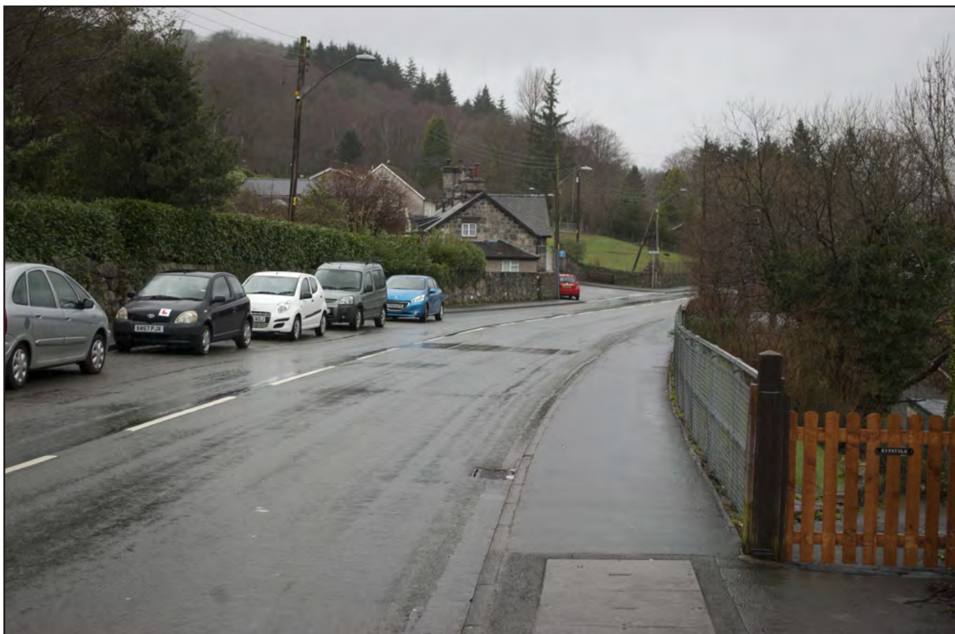
Plate 15: Section C-D: View west along street showing pipe route in pavement, showing former entrance to Bryngwyn
