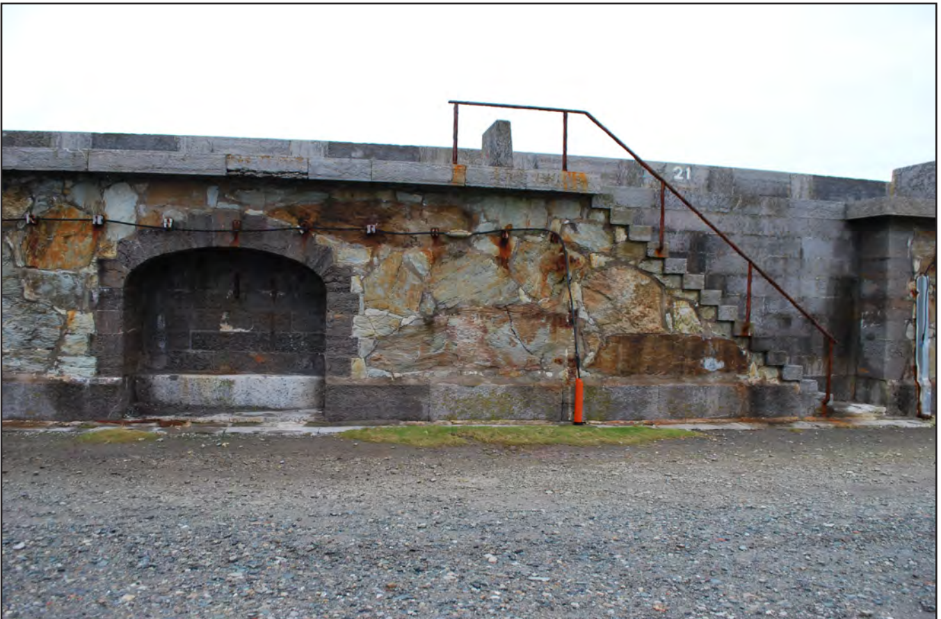
Plate 22: Holyhead Breakwater - view from south of refuge within the breakwater parapet and stairway between upper and lower levels (archive image: G2498_015).
