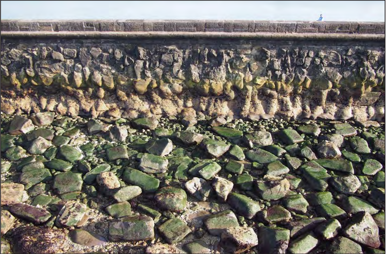
Plate 05: Seaward side view of rubble sourced from Holyhead Mountain used as supporting foundations of the parapet (sourced from Civil Engineering Solutions: 20150928 Holyhead Breakwater 186.jpg).
