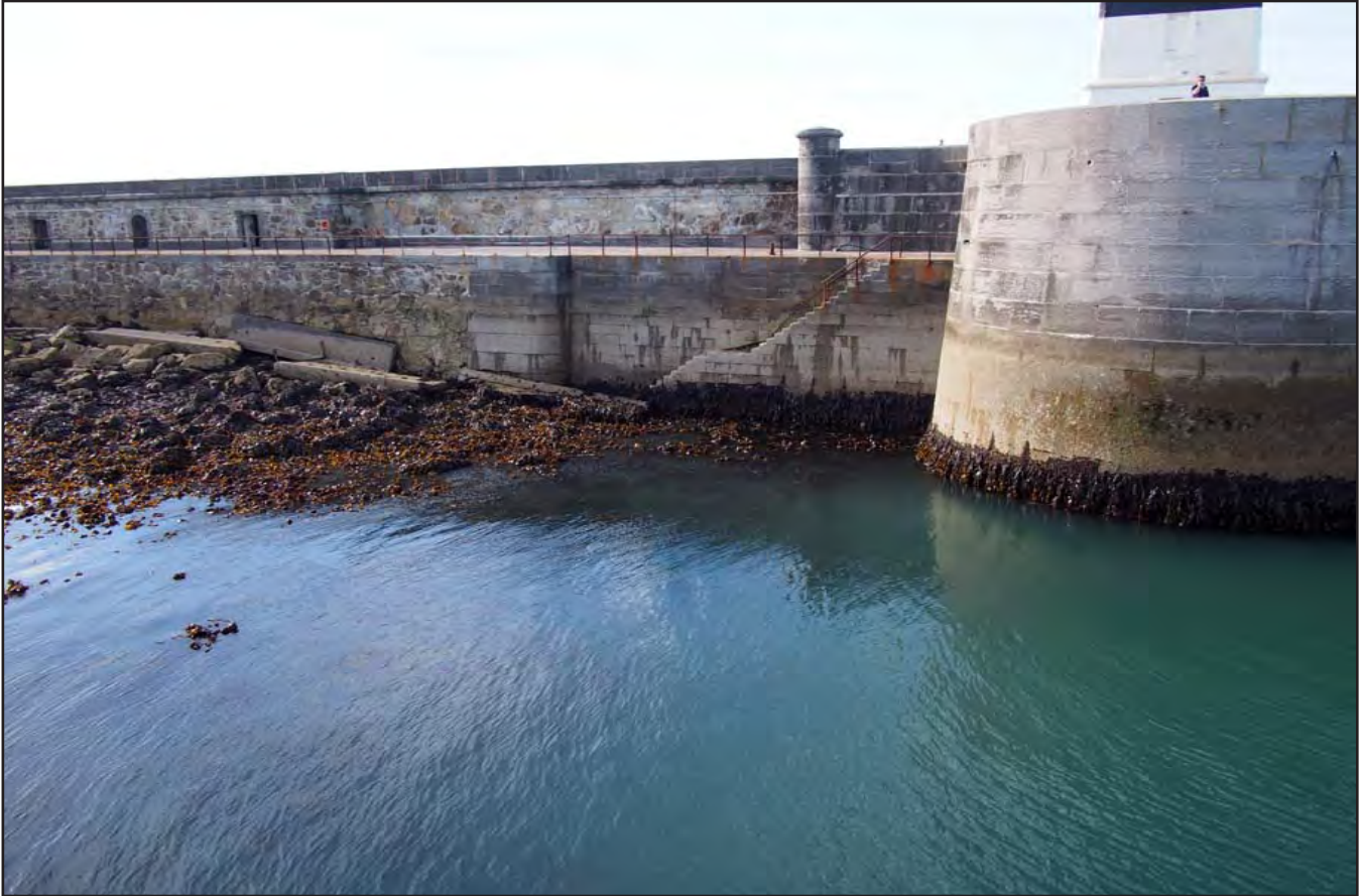
Plate 11: Portside view of the tail end of breakwater showing relationship with the ashlar masonry with view former storage and convenience area (sourced from Civil Engineering Solutions: 20150928 Holyhead Breakwater 151.jpg).
