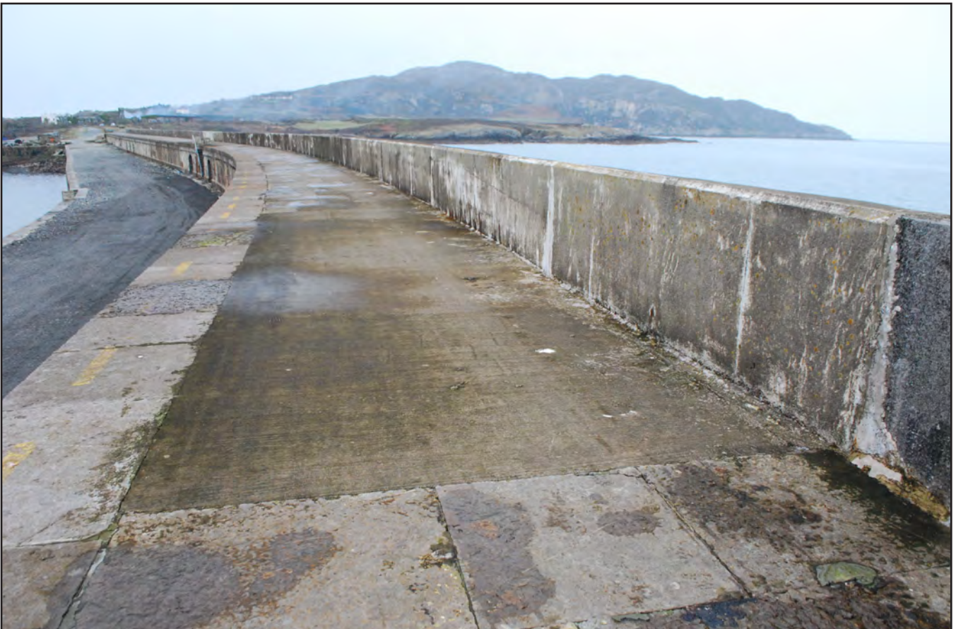
Plate 28: Holyhead Breakwater - view from east of storm damage repair to the parapet and carriageway (archive image: G2498_046).
