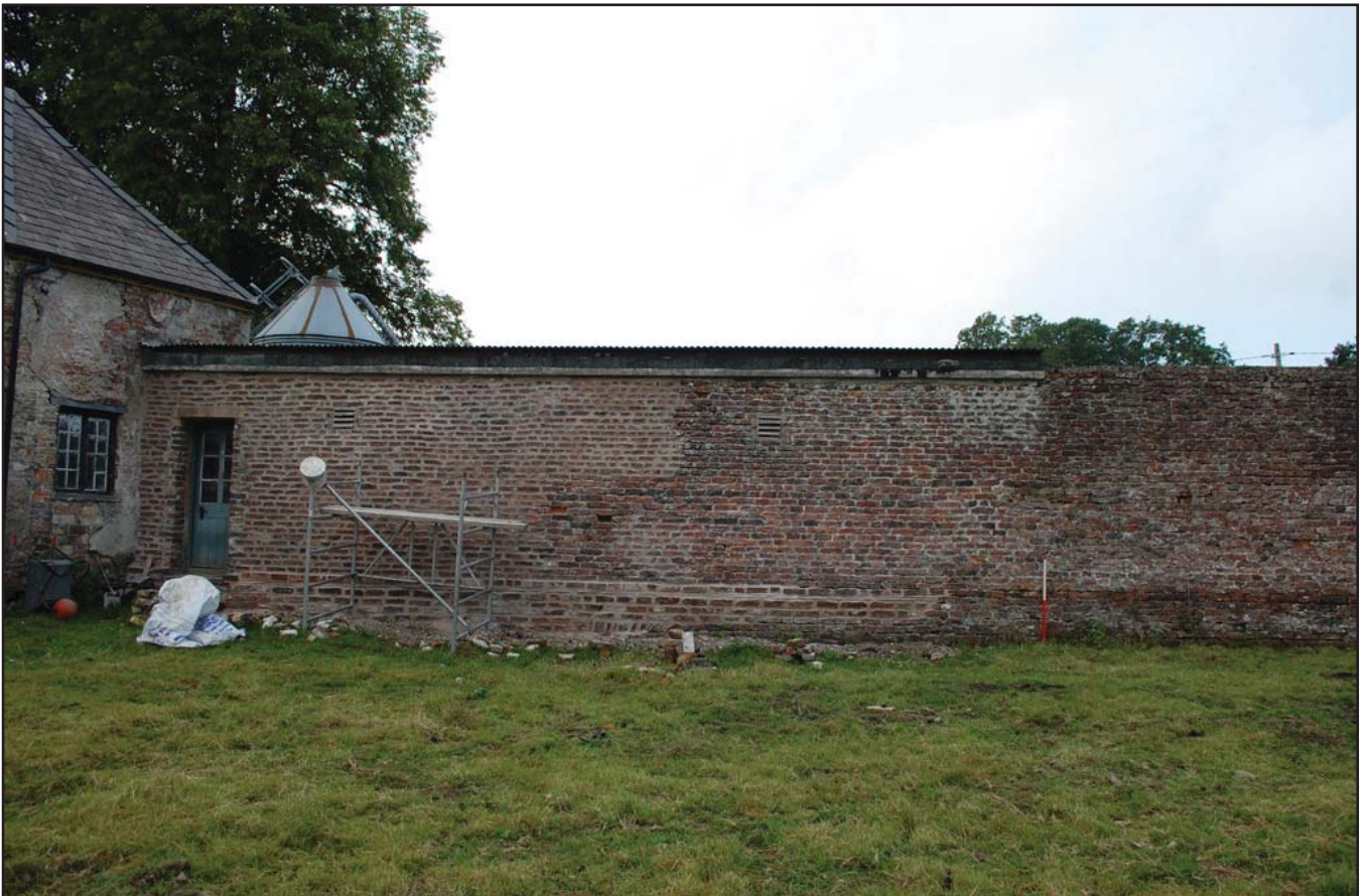
Plate 06: Re-built section of the southern wall. Scale 1m, viewed from the north-east.
