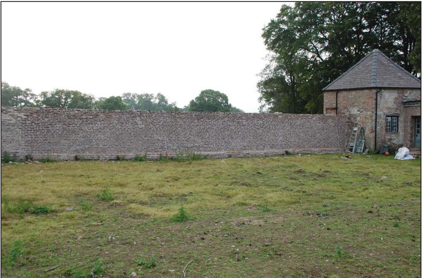
Plate 02: The eastern wall of the walled garden. Scale 1m, viewed from the north-west.
