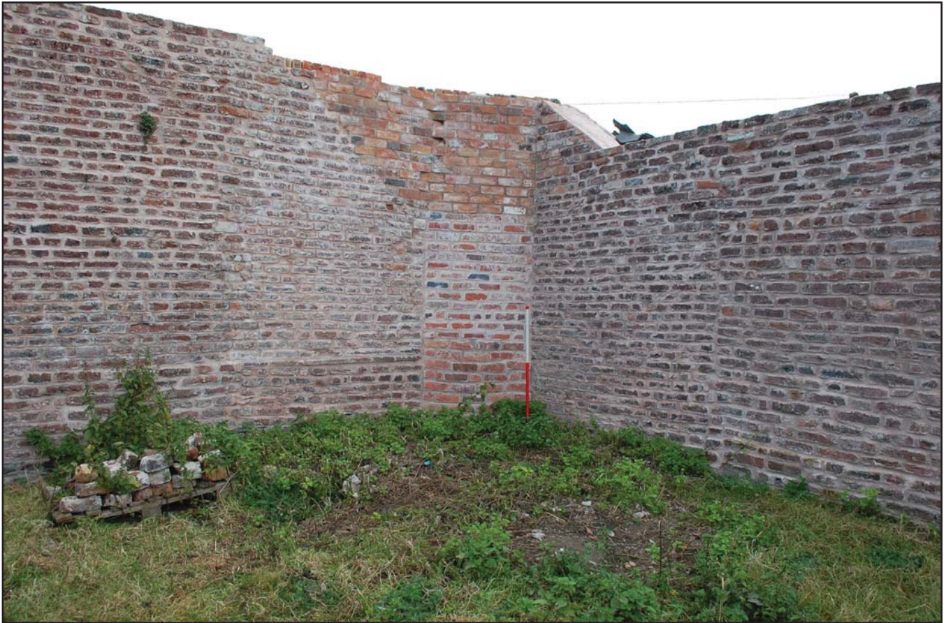
Plate 01: The northern & eastern walls of the walled garden. Scale 1m, viewed from the north-west.
