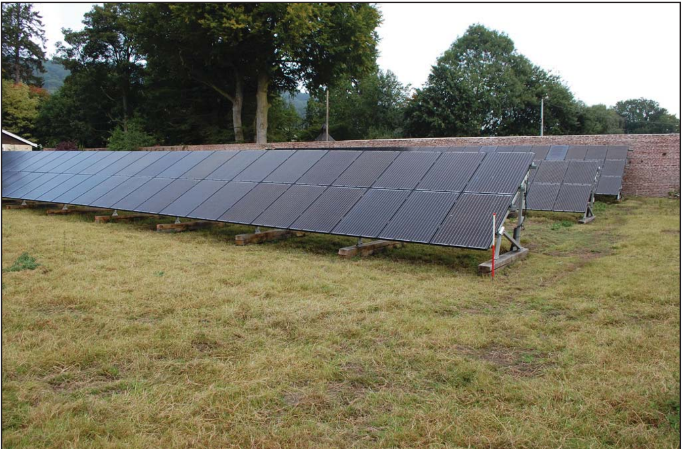
Plate 10: Solar panels at eastern end of the walled garden. Scale 1m, viewed from the south-west.
