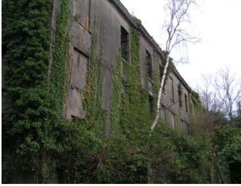
Buildings with vegetation growing within
