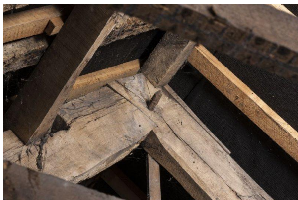
Figure 10 - Pegged apex to roof truss in chamber DS2014_112_024 (Crown Copyright. All rights reserved)
