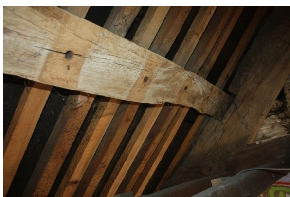
Figure 9 - Peg holes and shadowing for pegged rafters DS2014_285_020 (Crown Copyright. All rights reserved)
