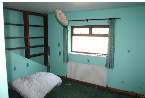
Figure 20 - Rear bedroom showing original line of catslide roof DS2014_285_025 (Crown Copyright. All rights reserved)
