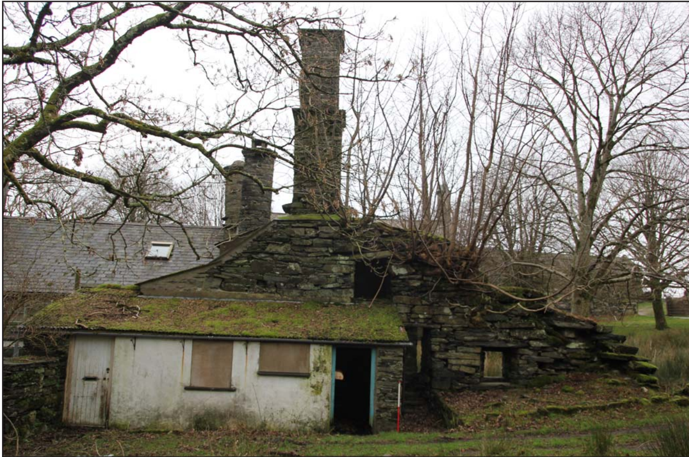
Plate 03: Parc 2 gable wall and 20th Century lean-to extension, from the northeast. Scale 1.0m.
